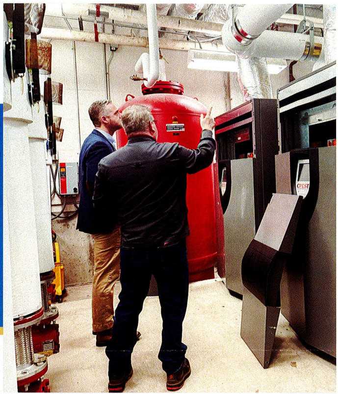
Harkness Center's lead custodian Robert Stoberl shows Dr. Michael Capuana, District Superintendent the newly installed boilers.
