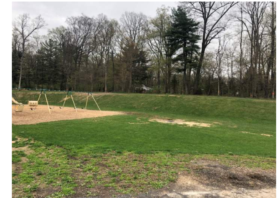
View of south side of playground area, showing hillside and secondary storm grate
