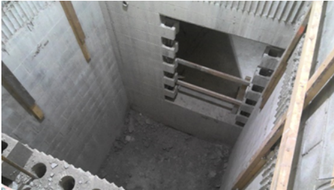
The new freight elevator in the cafeteria. Photo by Mr. Cooper
