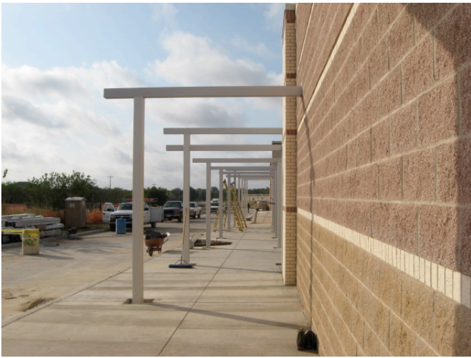
This is a view of the paving and canopy installation along the east wall of the two new additions to the building.
