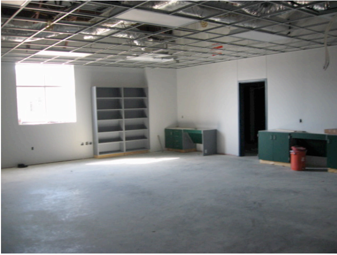
This is a view of one of the Science classrooms as cabinets and ceiling grid installation is nearing completion.
