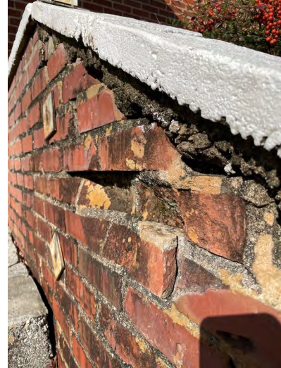
Masonry stairs in failure
