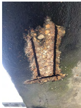
Exposed re-bar canopy
