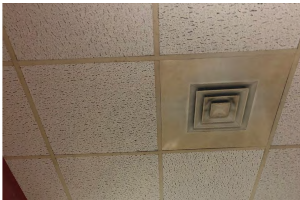
Aged and discolored ceiling grid
