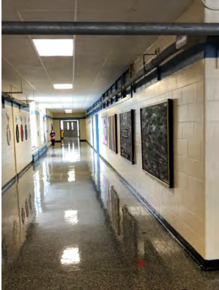
Hydronic and other exposed piping
