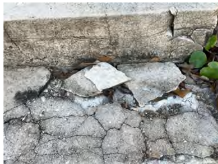
Concrete in failure
