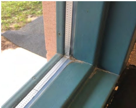
Broken seals on windows
