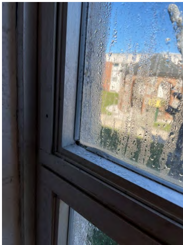
Window in failure
