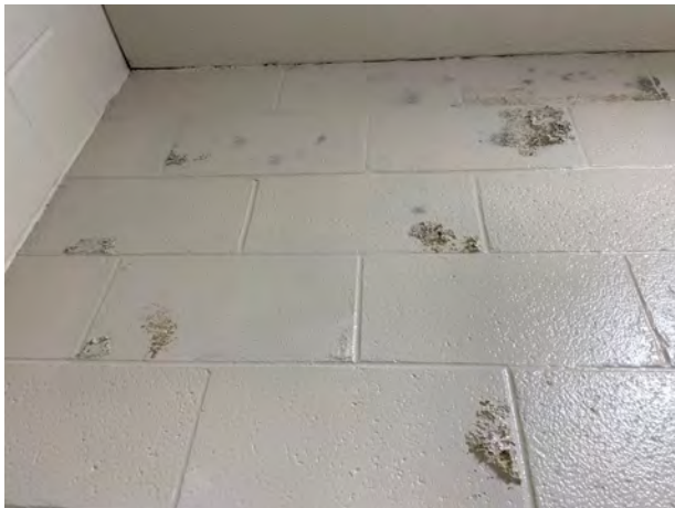
Spalling paint - water infiltration
