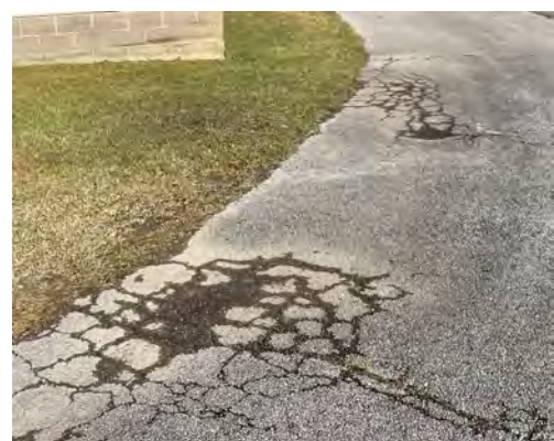
Asphalt in Failure
