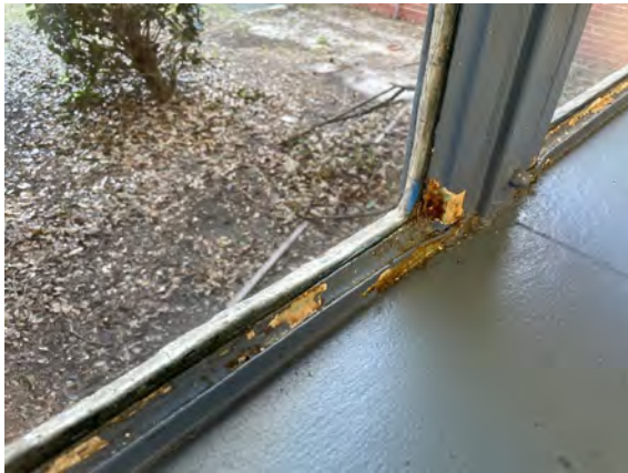
Windows in failure
