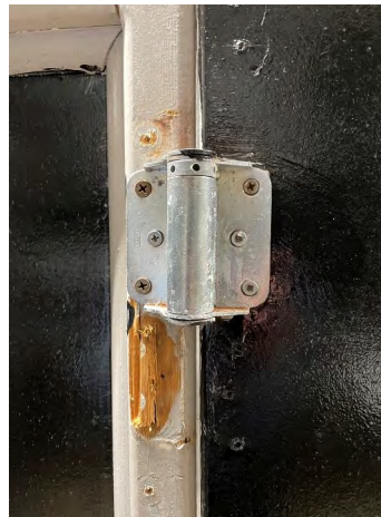
Hardware in failure
