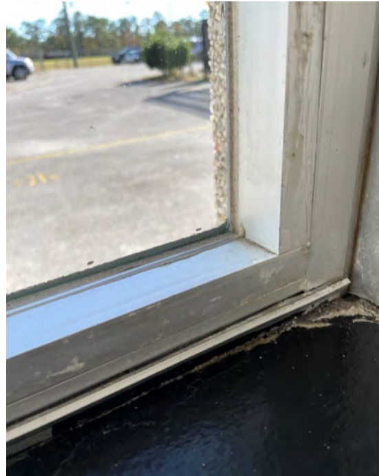
Old single pane non-insulated windows
