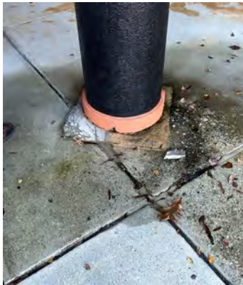
Concrete in Failure
