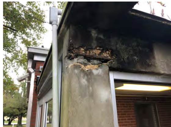
Concrete spalling at canopy
