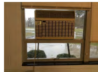
Window Unit - Supplemental Air Conditioning
