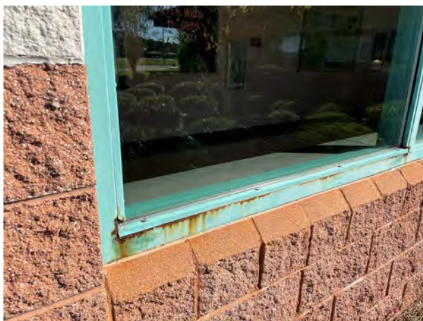
Window Frames in failure
