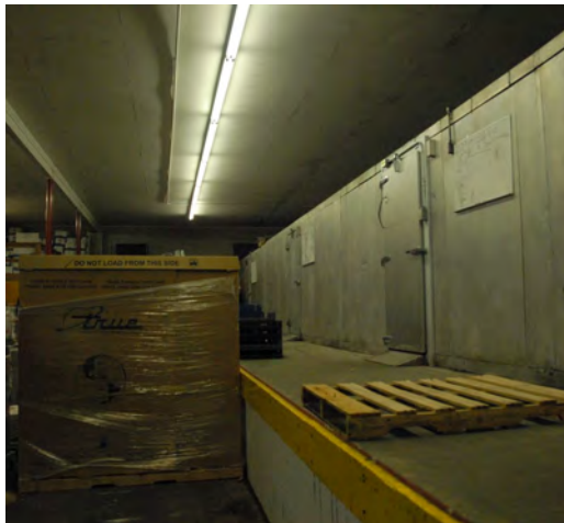
Units on Pad
