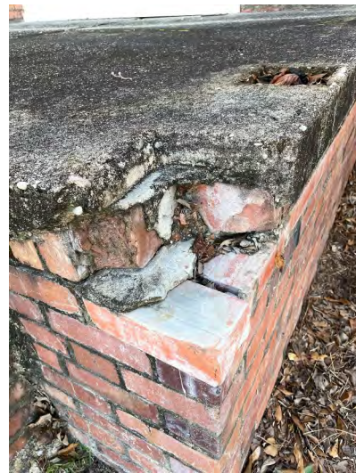
Brick stoop failure
