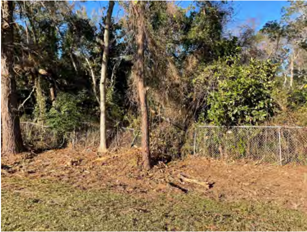
Fence at track in failure
