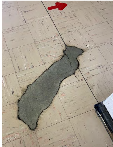
Floor Tile in Failure
