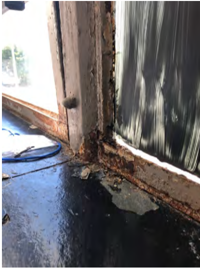
Window in failure
