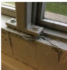
Fractured Sill and Block at Cafeteria
