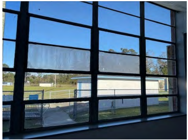
Old single pane non-insulated windows
