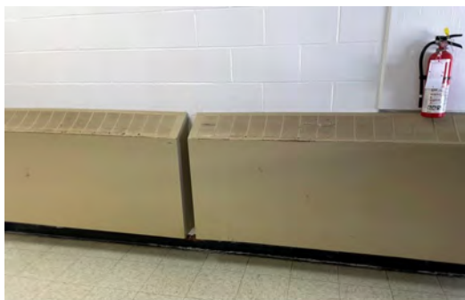
Aged HVAC System
