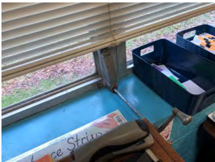
Old non-insulated windows
