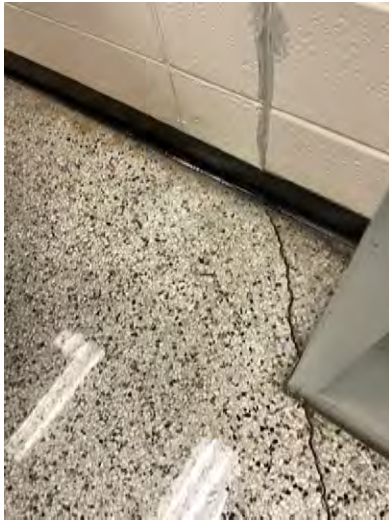
Floor Settlement - Sci Room
