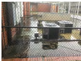
Drainage issues campus wide - Mechanical Units
