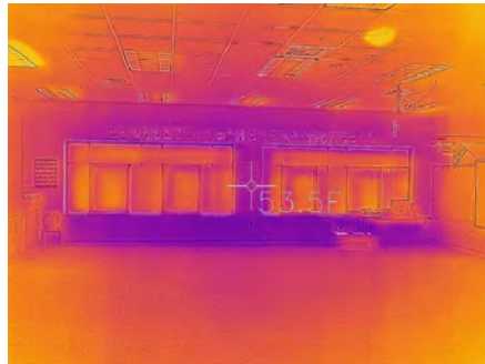
Thermograph of broken seals
