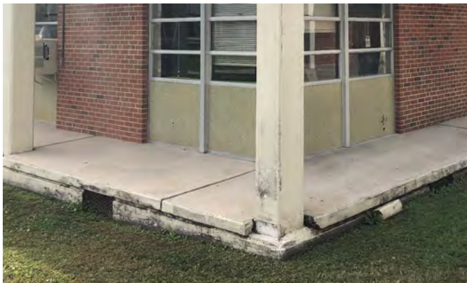
Concrete in failure
