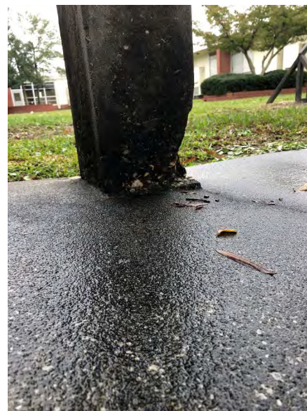
Concrete Column spalling
