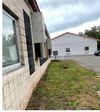
Wall Mounted HVAC Equipment
