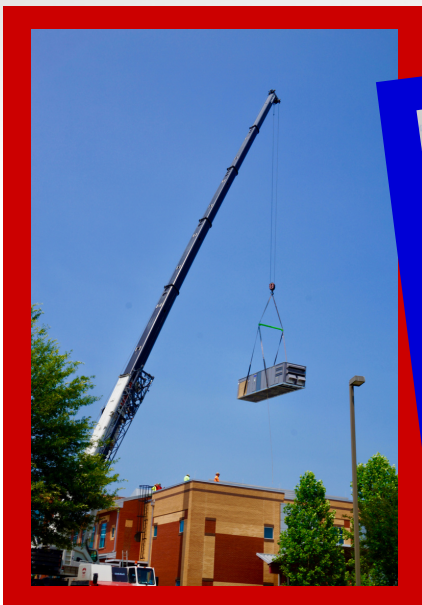
HVAC at Oconee County High School and North Oconee High School
