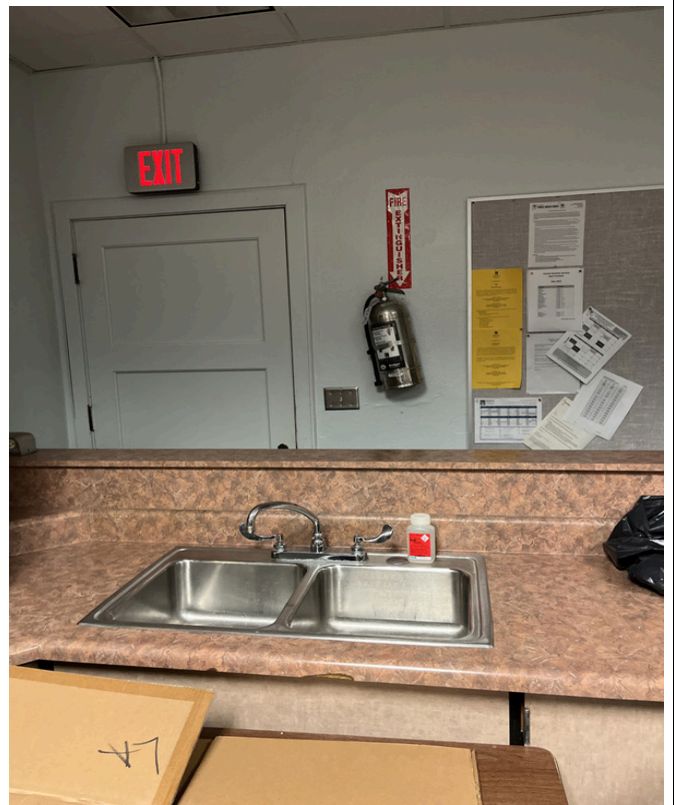
4/9/2024 - 2601-43 - Norclay Building - Room 828 - North Wall Right Sink
