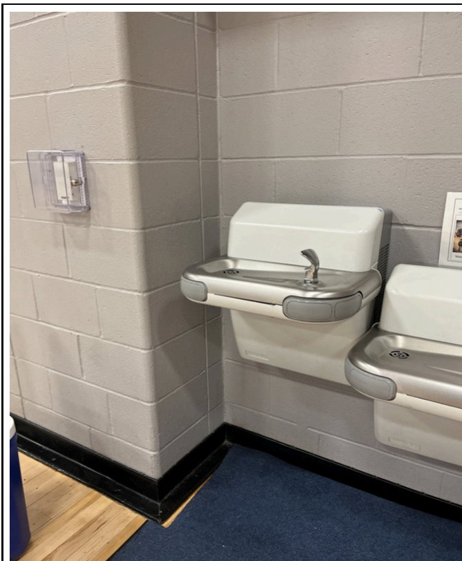
4/9/2024 - 2601-56 - Norclay Building - Gym - Left - Out of Order
