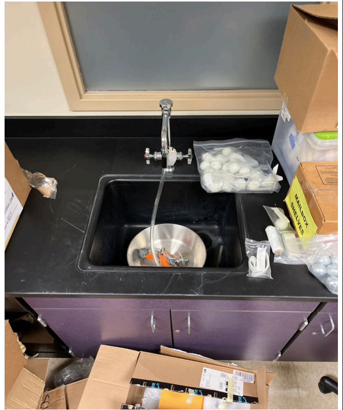
4/9/2024 - 2601-59 - Norclay Building - Room 817 Prep - Out of Order
