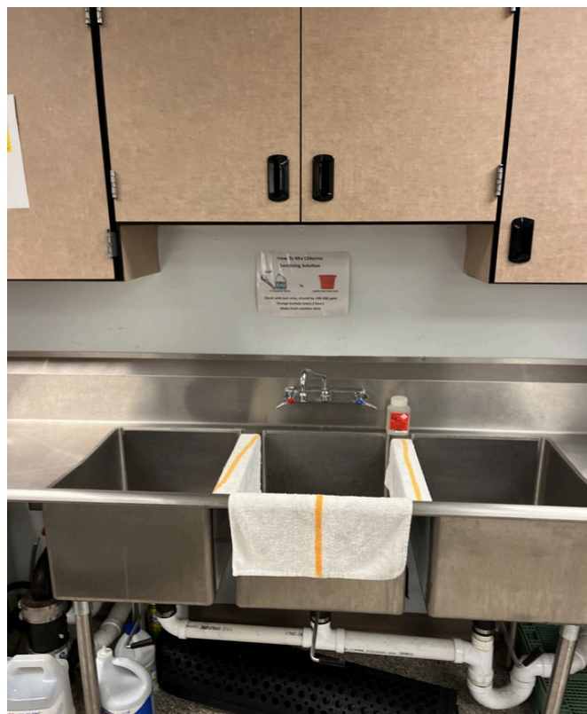
4/9/2024 - 2601-38 - Norclay Building - Room 828 - Southeast Sink
