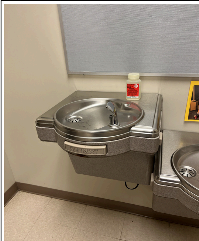
4/8/2024 - 221-23 - Nashua Elementary School- South Hall - Left Fountain
