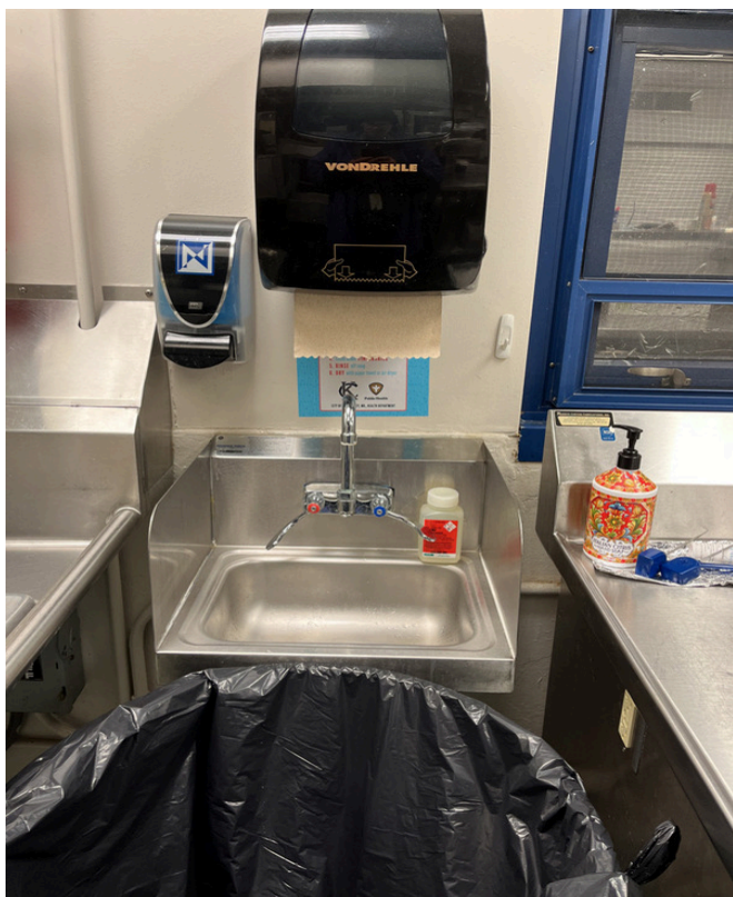
4/8/2024 - 221-7 - Nashua Elementary School- Kitchen - Northwest Handwashing Sink
