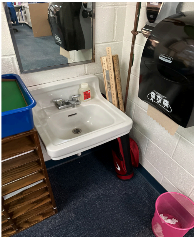
4/8/2024 - 221-19 - Nashua Elementary School- Room 12 - Handwashing Sink
