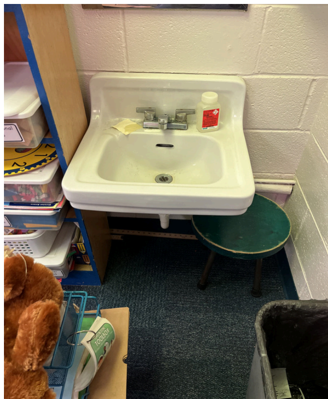
4/8/2024 - 221-15 - Nashua Elementary School- Room 8 - Handwashing Sink
