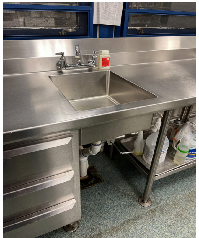
4/8/2024 - 221-8 - Nashua Elementary School- Kitchen - North Sink
