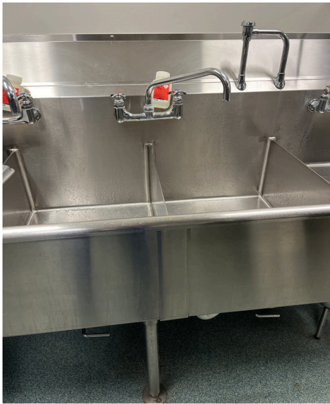
4/8/2024 - 221-5 - Nashua Elementary School- Kitchen - Middle Sink
