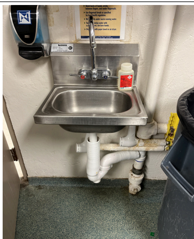
4/8/2024 - 221-2 - Nashua Elementary School- Kitchen - Handwashing Sink
