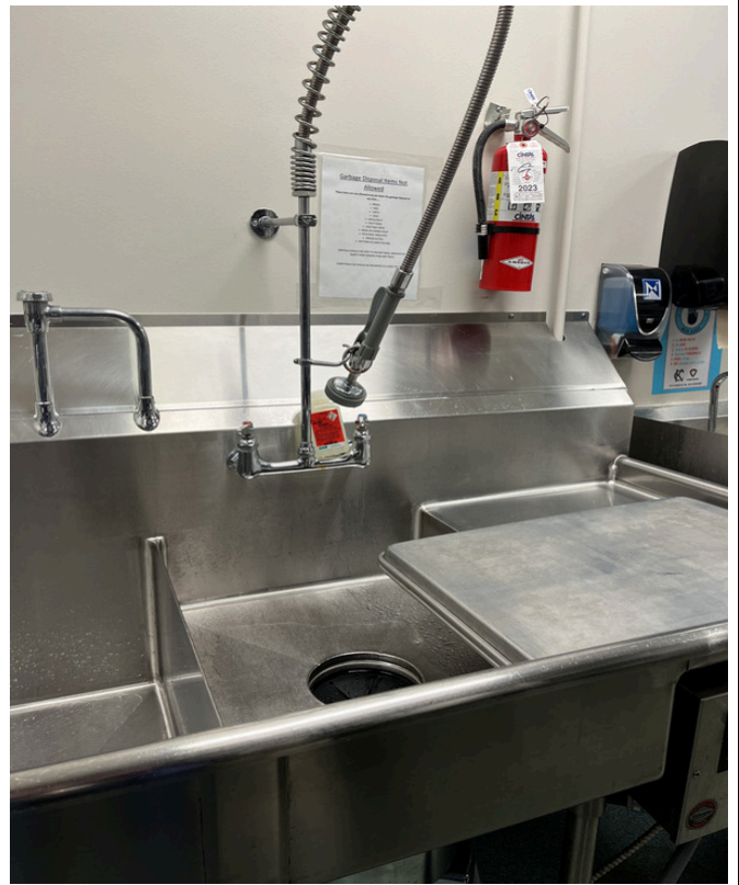
4/8/2024 - 221-6 - Nashua Elementary School- Kitchen - Northeast Sink
