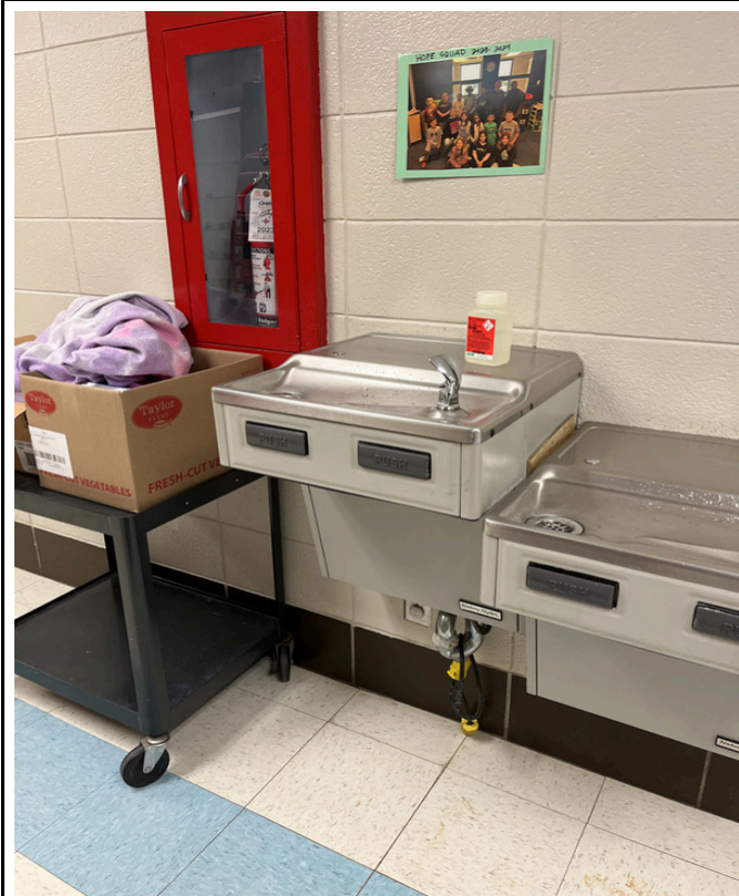
4/8/2024 - 221-25 - Nashua Elementary School- North Hall - Left Fountain
