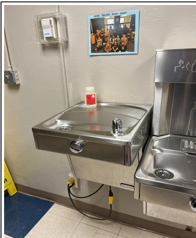
4/8/2024 - 221-9 - Nashua Elementary School- Cafe Drinking Fountain - Left Fountain
