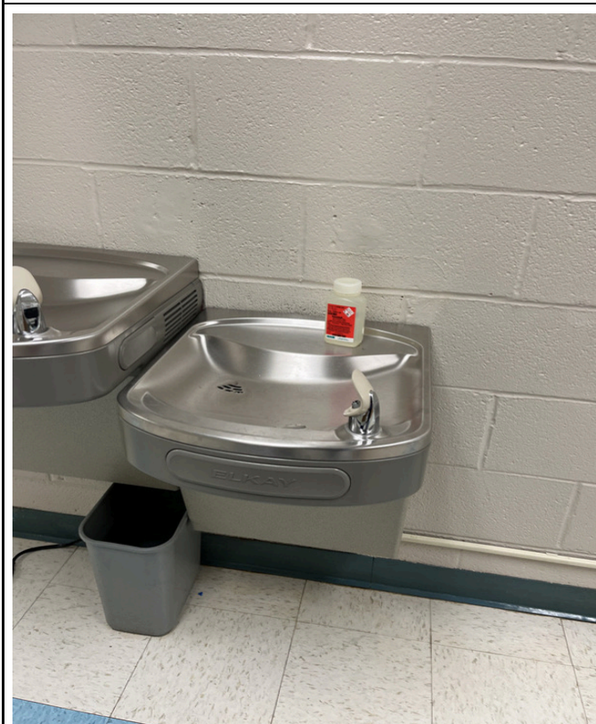
4/8/2024 - 221-17 - Nashua Elementary School- Drinking Fountain - Right
