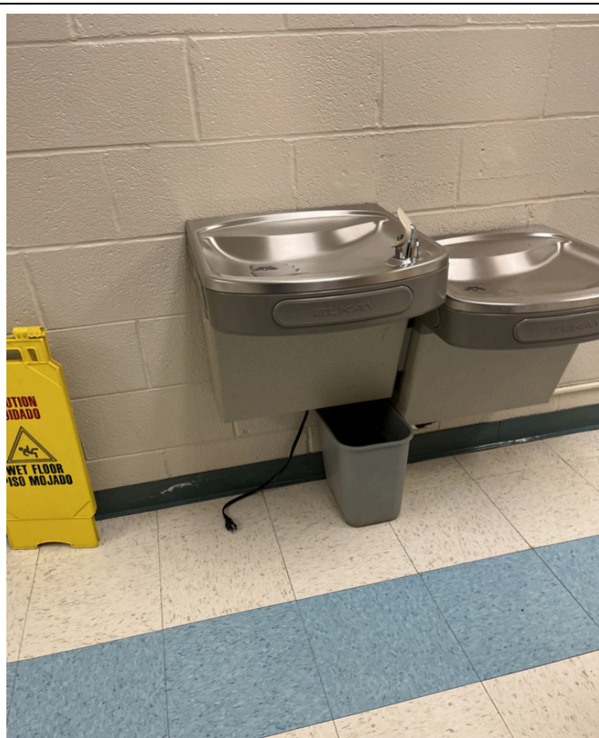
4/8/2024 - 221-29 - Nashua Elementary School- Drinking Fountain - Left
