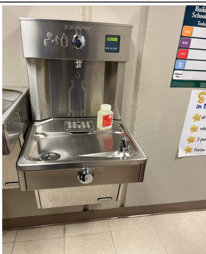
4/8/2024 - 221-10 - Nashua Elementary School- Cafe Drinking Fountain - Right Fountain
