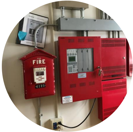
Replace Fire Alarms
