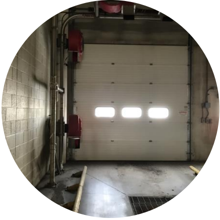
Exhaust Ventilation At Cleaning Bay
