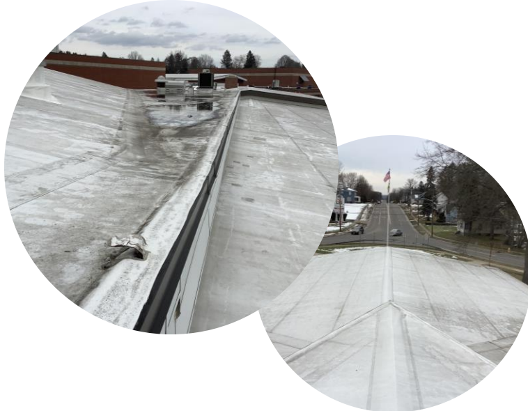
Replace Out of Warranty Roofs – 22 Years Old
