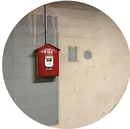
Replace Fire Alarm System, 20+ Years Old
