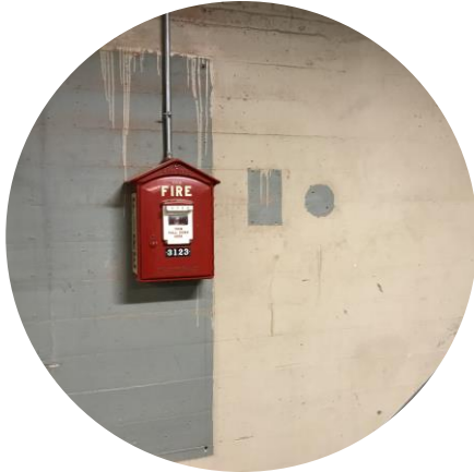
Replace Fire Alarm System, 20+ Years Old
