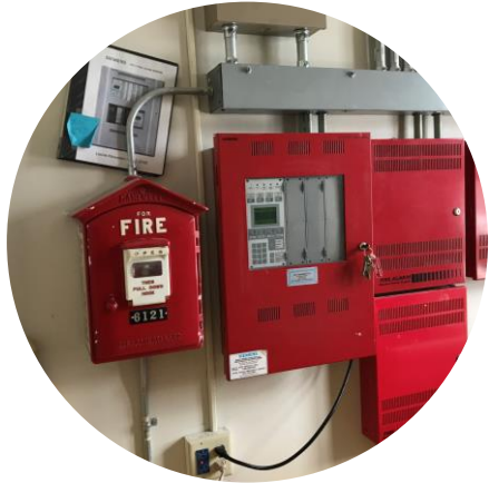
Replace Fire Alarms
