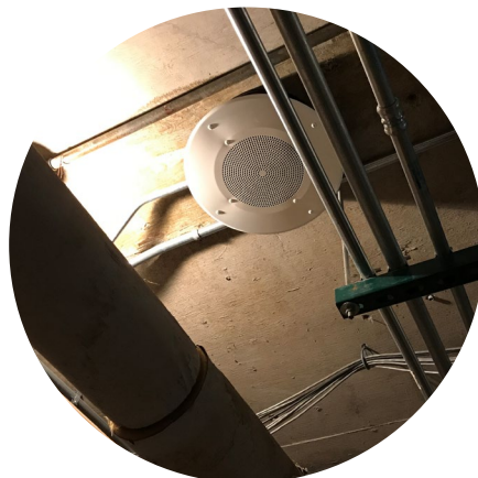
Building Wide PA System
