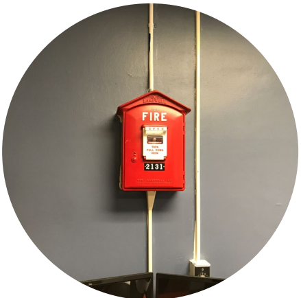
Provide Code Compliant Fire Alarm System
