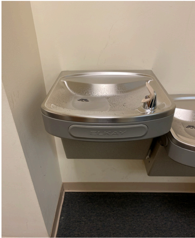
3/12/2024 - 9600-1 - ECC - 003782B-Next to 408-Left
