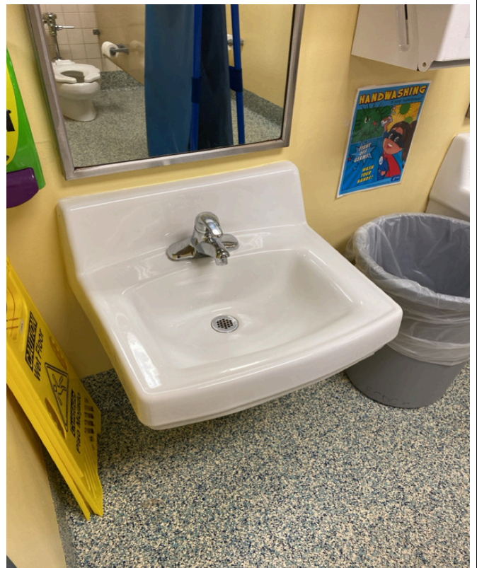
3/12/2024 - 9600-20 - ECC - 002031-Between 205-206-Left
