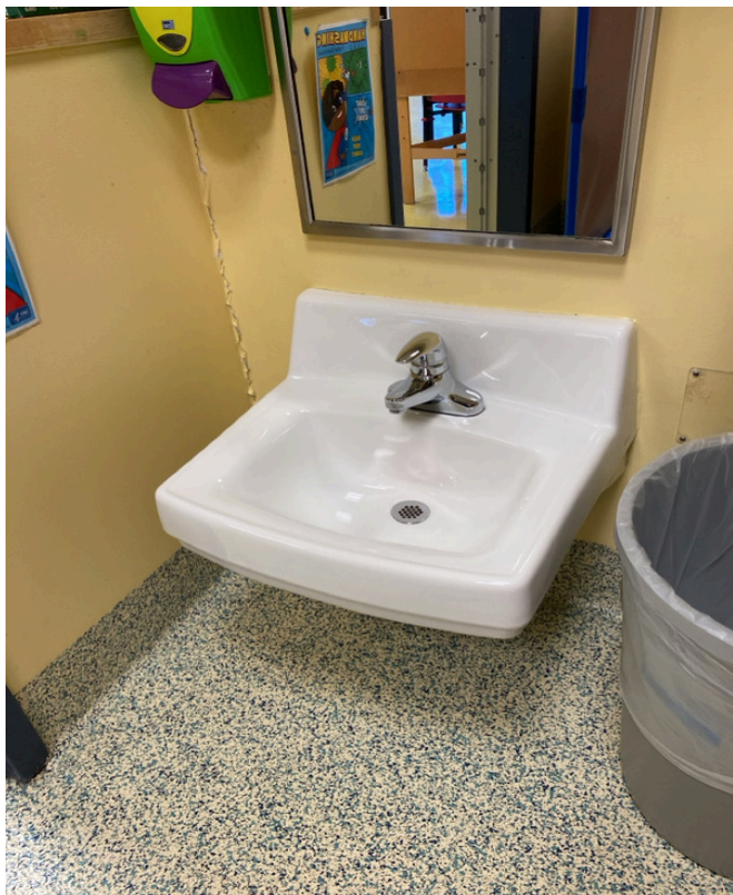
3/12/2024 - 9600-15 - ECC - 002026-Between 201-203-Left
