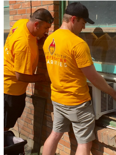
In collaboration with Commissioner Roy Brooks Precinct 1 Tarrant County, and Fort Worth Fire Department, A/C units were donated and installed for those in need.
