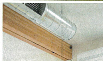
HVAC provides clean, healthy air.
