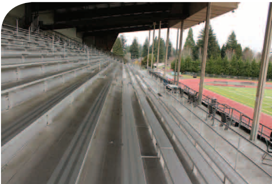
The District Stadium has new aluminum and steel bleachers in the upper seating area. Replacing the 26-year-old wood seating, these new long-lasting seats will provide safer seating for years to come.
