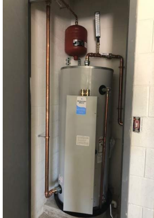
05.14.24 - Water Heater at Concession Stand
