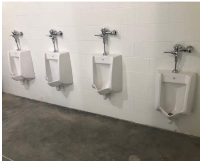
05.14.24 - Men's Restroom Toilet Fixtures
