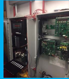
Main Control Panel Installed
