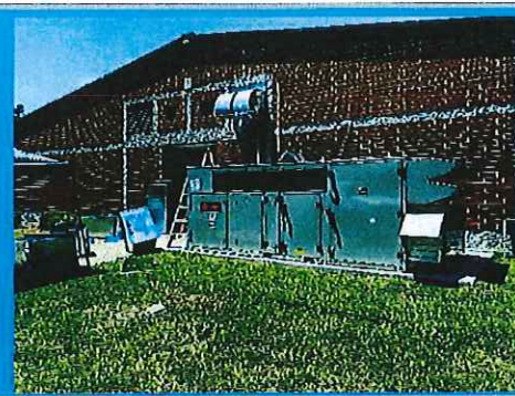
SSE New Units Connected
