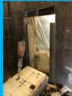
Return Air - Wall Penetration
