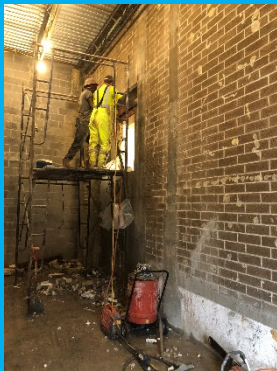
Supply Air - Wall Penetration
