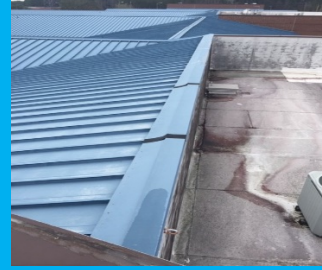
Parapet Metal Cap to be Replaced
