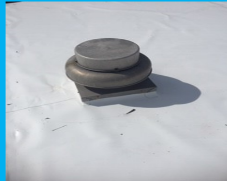
Temporary Flashings around vent
