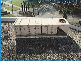
Existing Makeup Air Unit (MAU)
