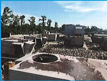
Old Roof-Top Units (RTUs)
