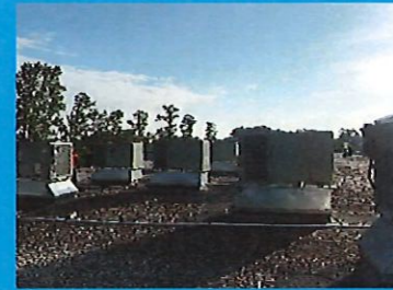
New RTUs installed
