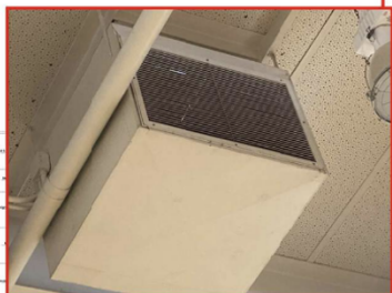
Daylight visible through damper
