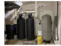
Water softener tanks
