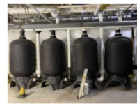
In-line chlorination tanks
