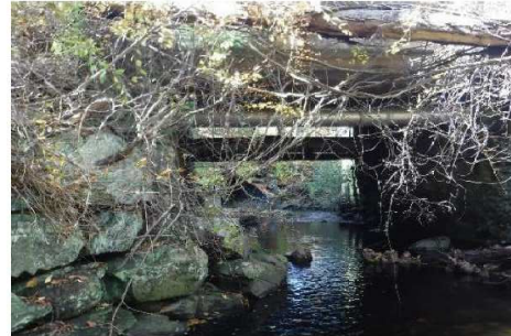
Photo 17: Overgrowth and voids at the northwest wingwall
