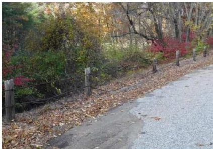
Photo 12: Broken cable and missing post at the northwest approach railing
