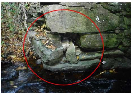
Photo 16: Partial abutment collapse at the northwest abutment corner due to undermining
