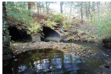
Photo 18: Restricted waterway due to accumulation west of the bridge
