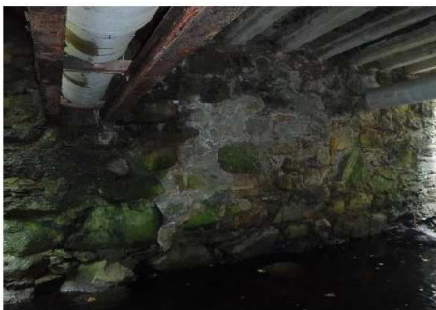
Photo 15: Minor voids and cracks in the north abutment
