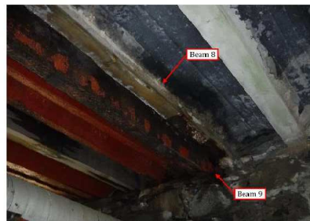
Photo 13: Severe deterioration to Beams 8 and 9
