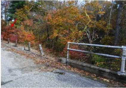
Photo 11: Loose cables and broken posts at the northeast approach railing
