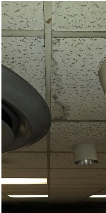
Photograph No. 2 Visible Mold Growth on Ceiling Tile - Room 29 (Sample T2 Location)
