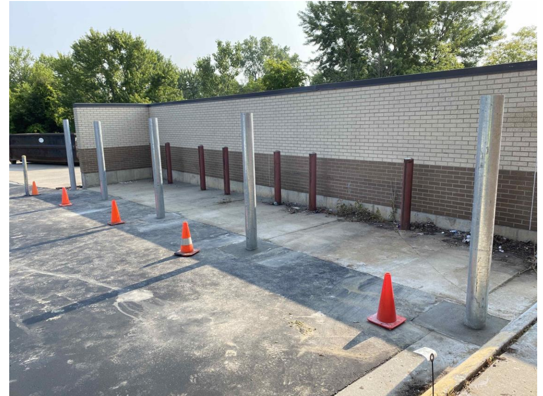
The dumpster gate existing bollards have been removed, and new bollards have been installed.
