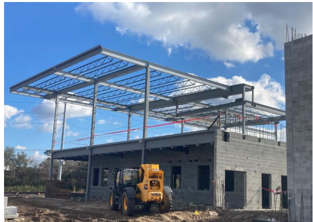
2 nd Floor Media Center Steel
