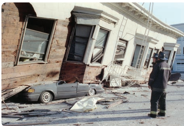
The 1989 earthquake in San Francisco caused the third floor of this apartment building to collapse onto this car.
