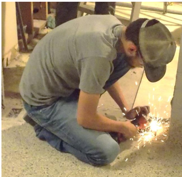
Masonry - Brad Pulver (B) is cutting metal conduit below the level of the floor.
