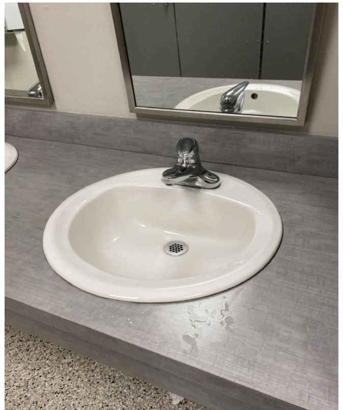
3/18/2024 - 650-18 - Epic Elementary - 001896-By 202-Girl's Restroom-Right
