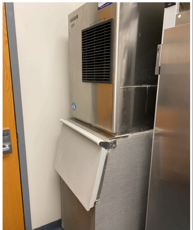
3/18/2024 - 650-44 - Epic Elementary - 002217- Kitchen
