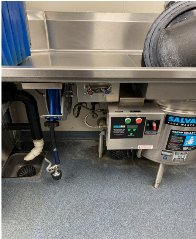
3/18/2024 - 650-49 - Epic Elementary - 004524- Kitchen
