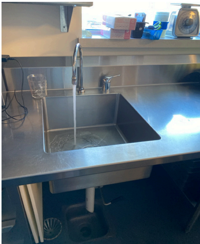
3/18/2024 - 650-47 - Epic Elementary - 004527- Kitchen
