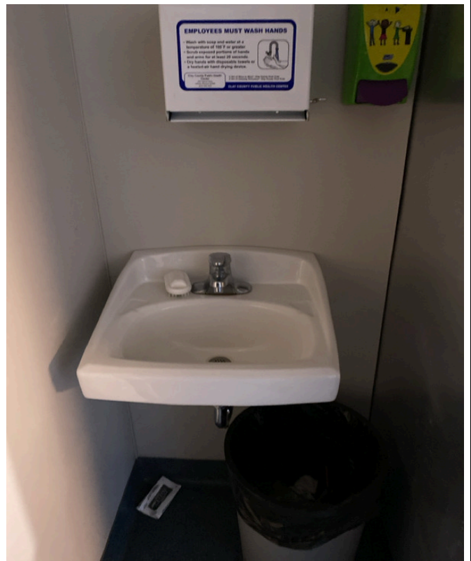
3/18/2024 - 650-48 - Epic Elementary - 004528- Kitchen
