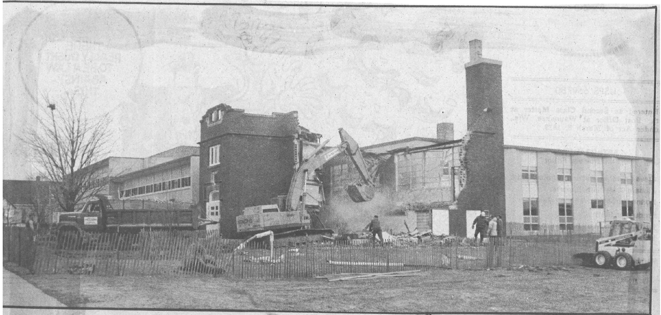
Construction workers for Melvin Paulson & Sons Inc. of DeForest began demolishing the Junior High Annex, formerly the old Waunakee Grade School, on Monday. A two-classroom addition is being planned for the site. Persons interested in obtaining bricks as mementos from the old annex can contact the Waunakee High School office. The bricks will be given away as long as the supply lasts. (Photo by Steve Kruschek)
