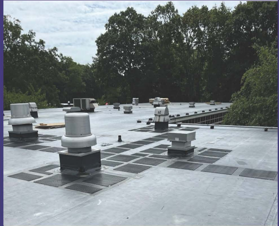
Roof Replacement & HVAC for HS Cafeterias and Auditorium to take place over Summer 2024
