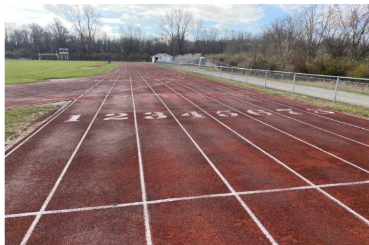
Worn and water damage track
