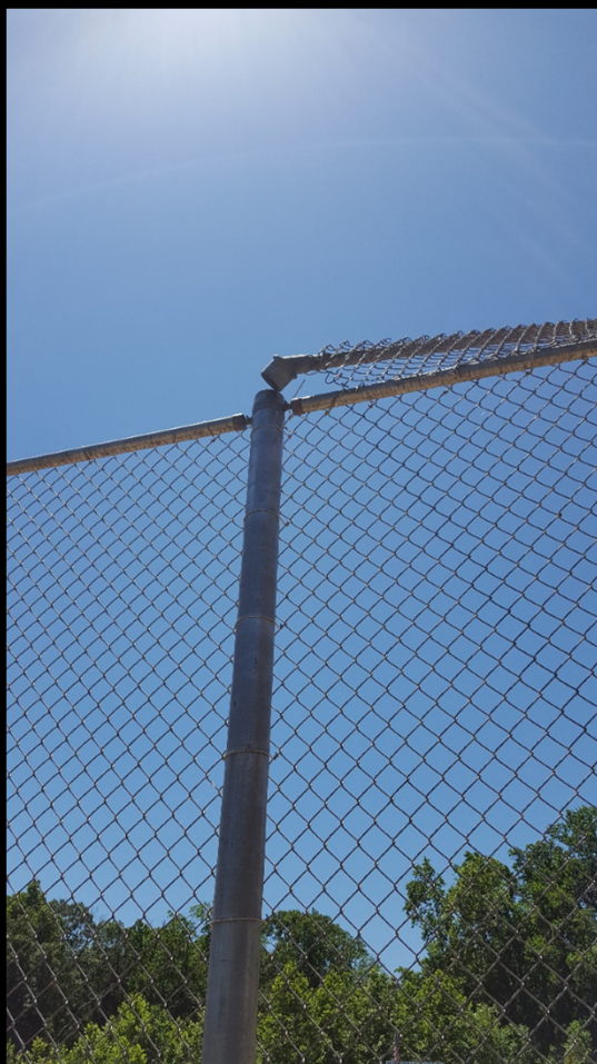
01. Backstop Needing Repair
