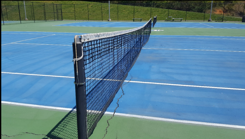
05. Net Post Foundation Heaving and Cracking
