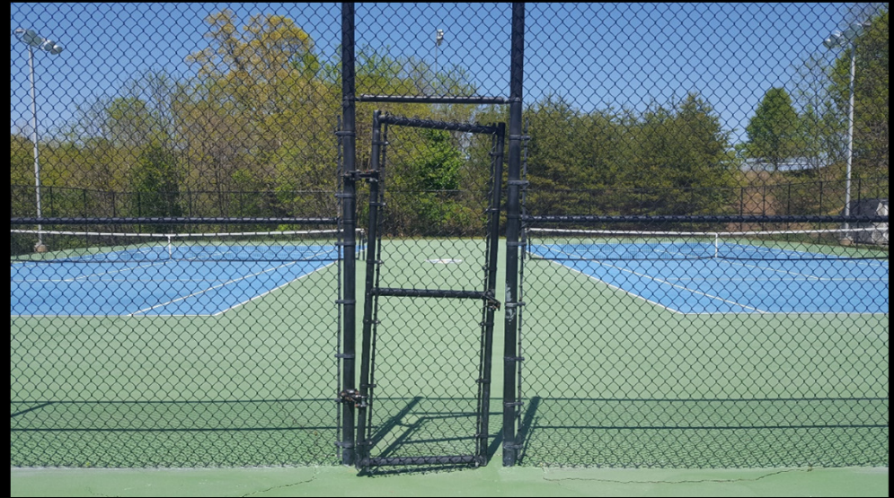
04. Entrance Gate Needs Replaced
