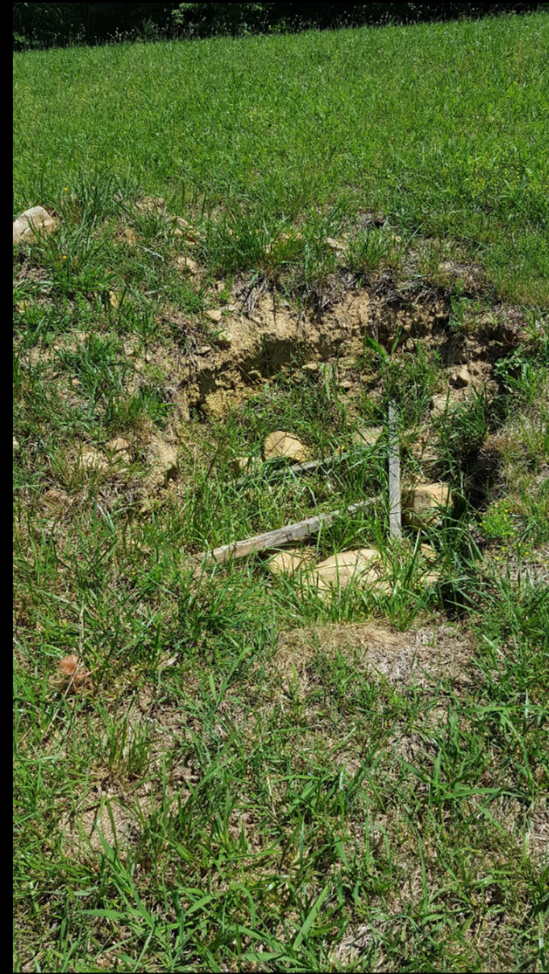
02. Sink Hole Outside Perimeter Fence
