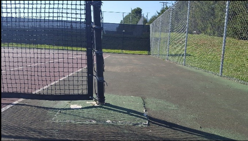
03. Net Post Foundation Heaving
