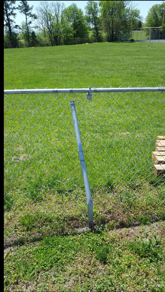
04. Perimeter Fence Needing Repair
