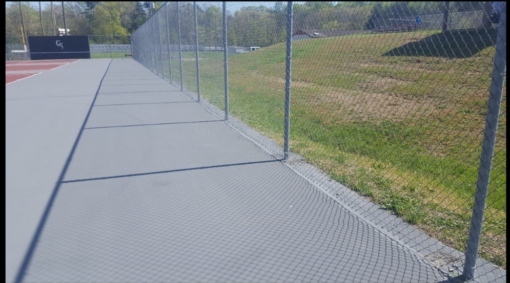
06. Perimeter Fence no Bottom or Mid Rail
