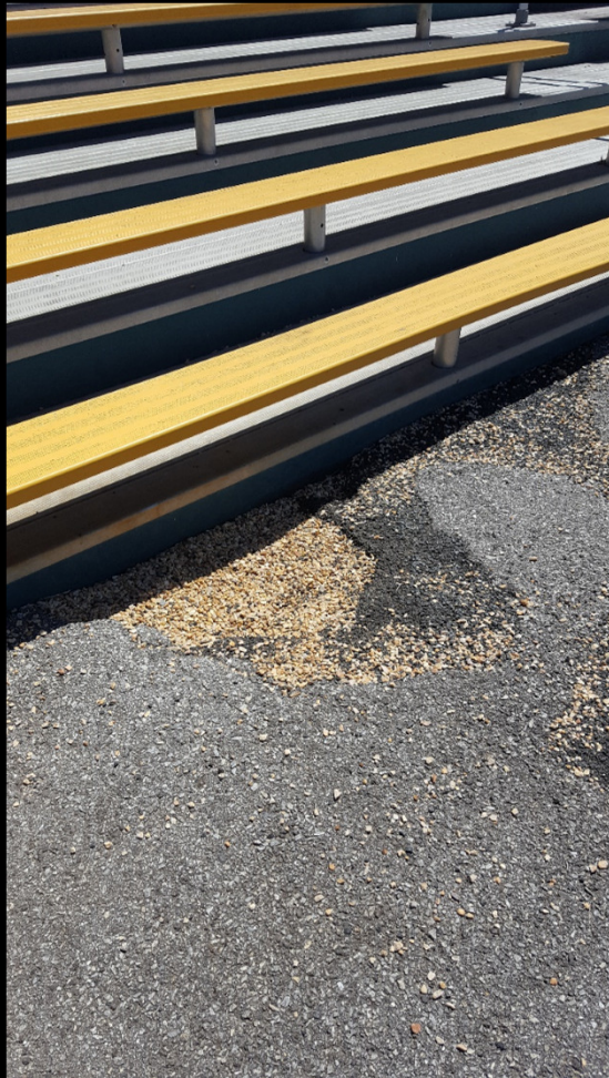
05. Wash Out at Visiting Bleachers
