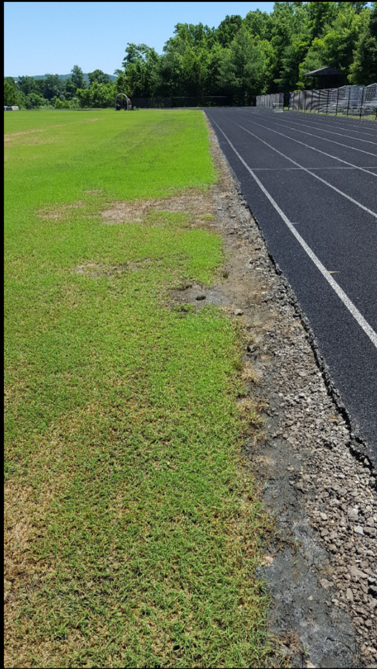
03. Water Ponding Along Edge of Track
