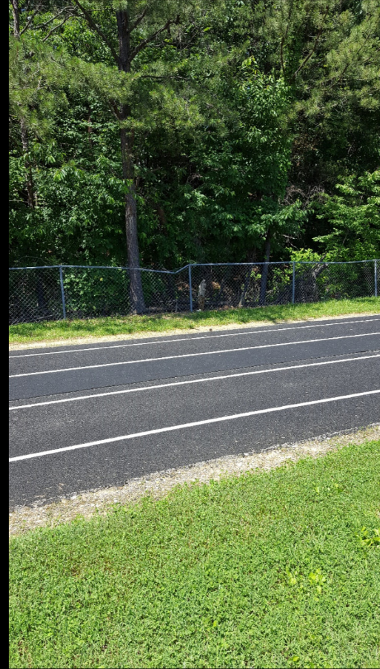
04. Damaged Perimeter Fence
