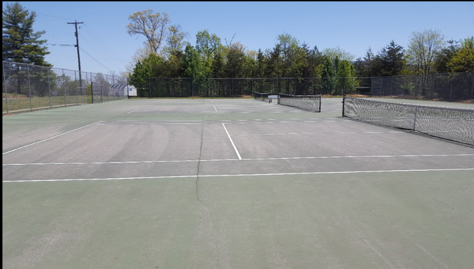
01. Surface Fading and Cracks
