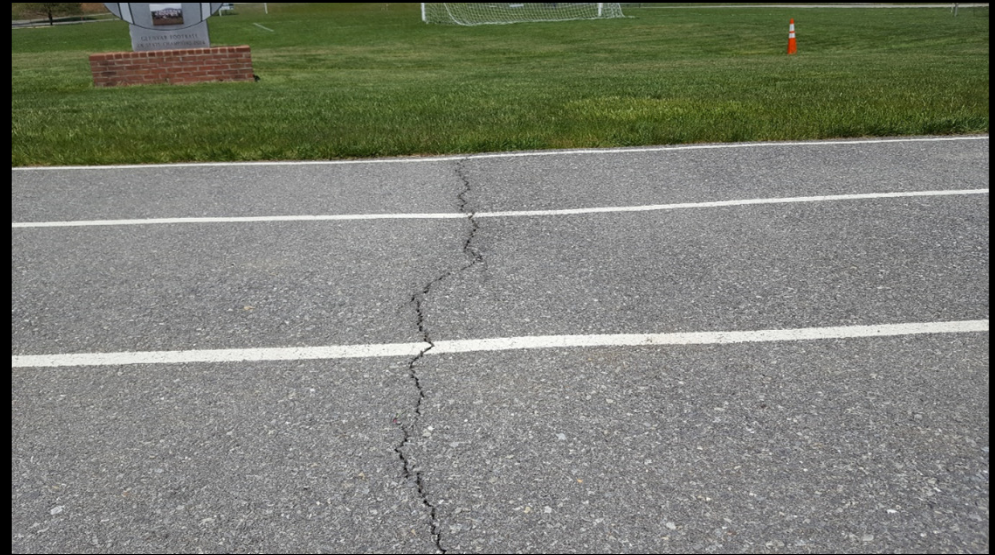
02. Crack in Asphalt
