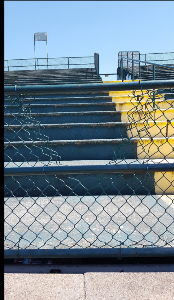
02. Bleacher Fence Needing Repair
