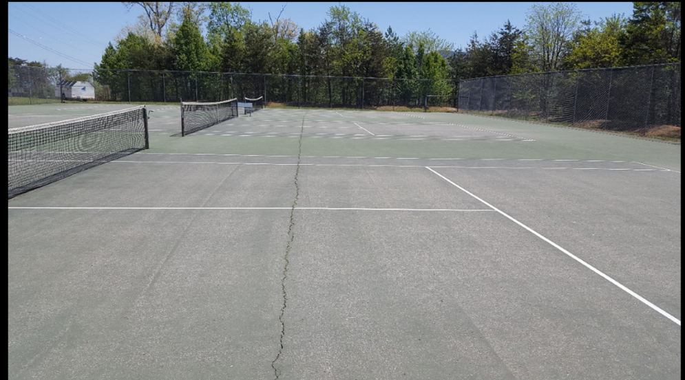
02. Surface Fading and Cracks
