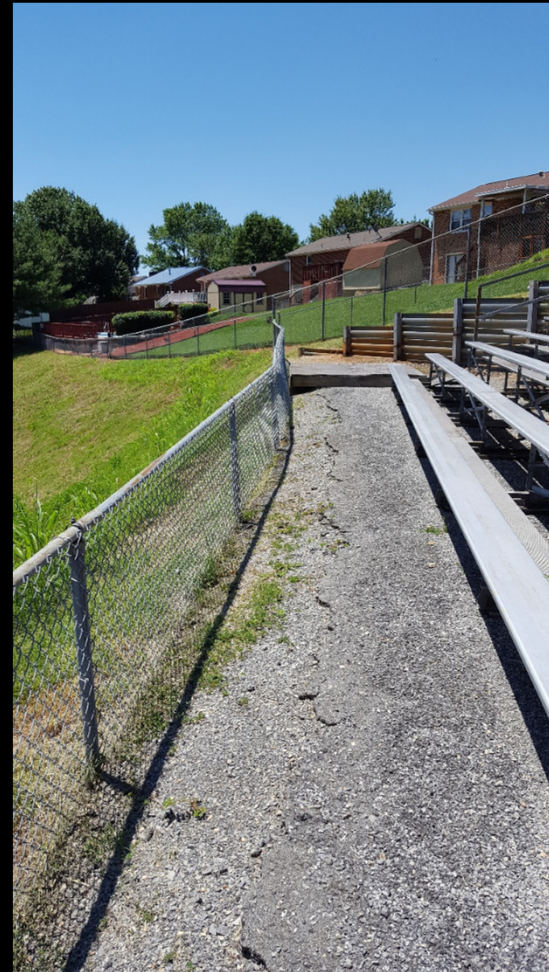
02. Upper Level Fence Sagging
