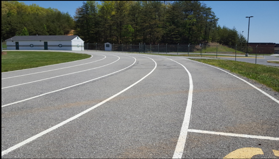
01. No Surfacing, Asphalt Only
