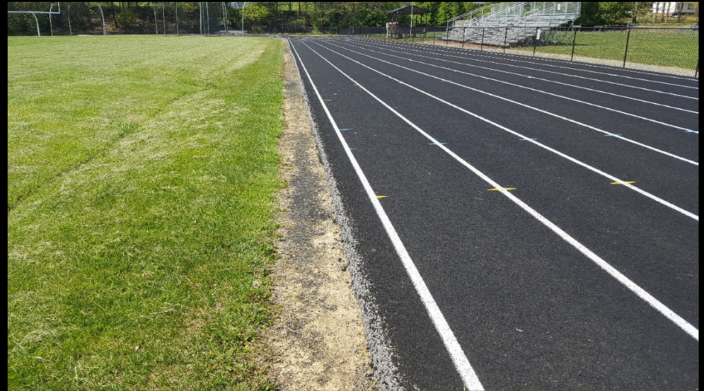
04. Track Edge Where Water Collects
