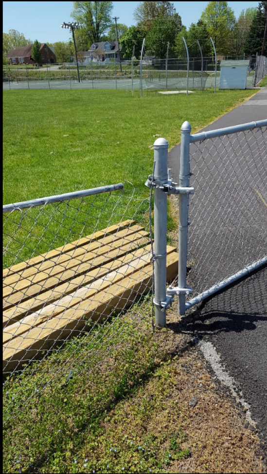
05. Perimeter Fence Needing Repair
