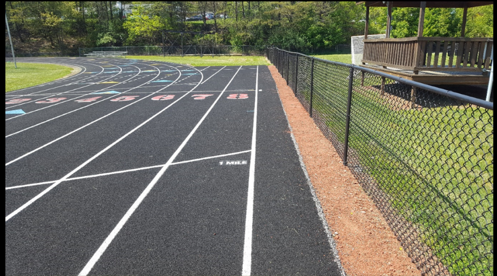
06. No Perimeter Curb
