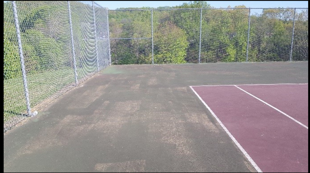
04. Areas of Delamination and Streaking
