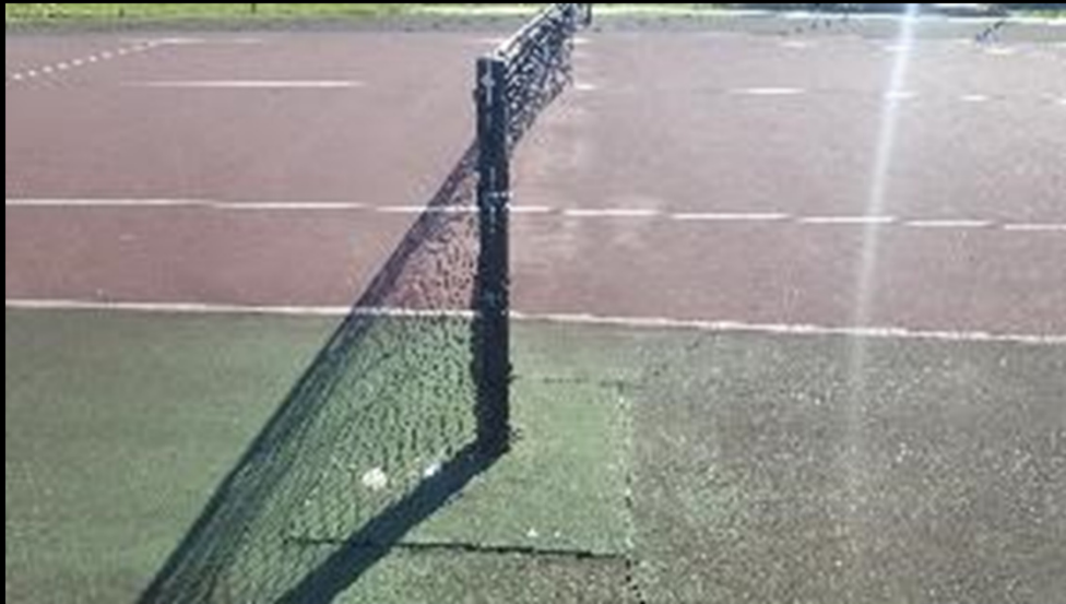
01. Net Post Anchor Heaving
