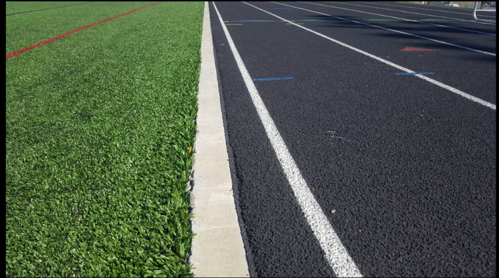
02. No Trench Drain
