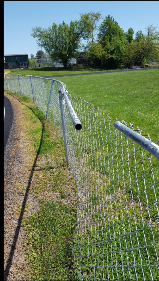
06. Perimeter Fence Needing Repair
