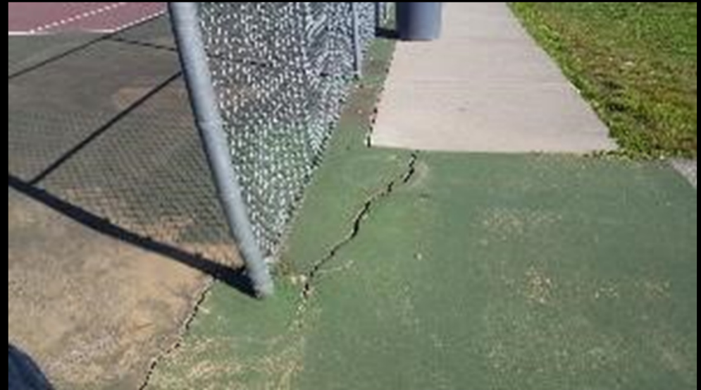
02. Crack at Northwest Corner Entrance
