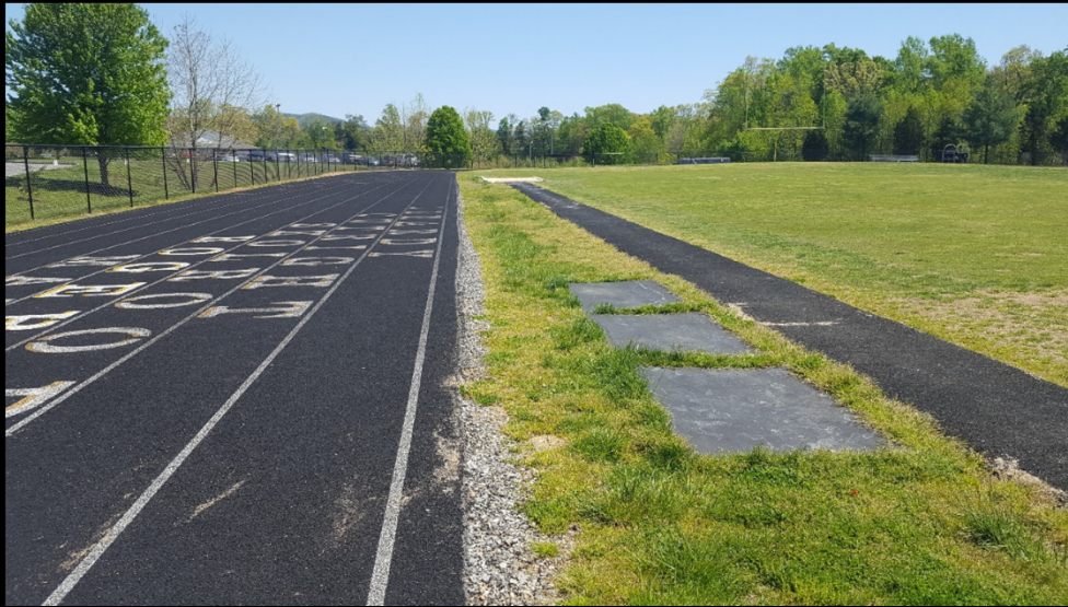
01. Exposed Inside Edge
