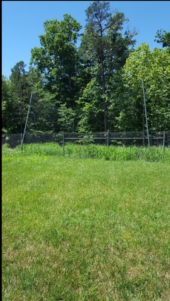
03. End Netting Needs Replaced
