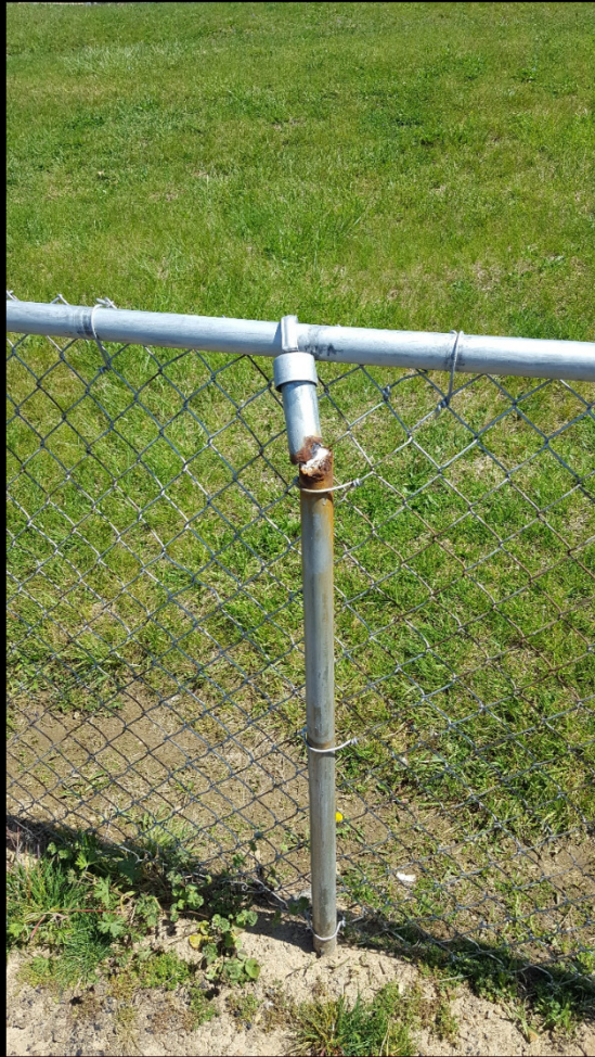
03. Perimeter Fence Needing Repair
