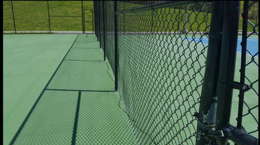
06. Fence Foundation Cracking
