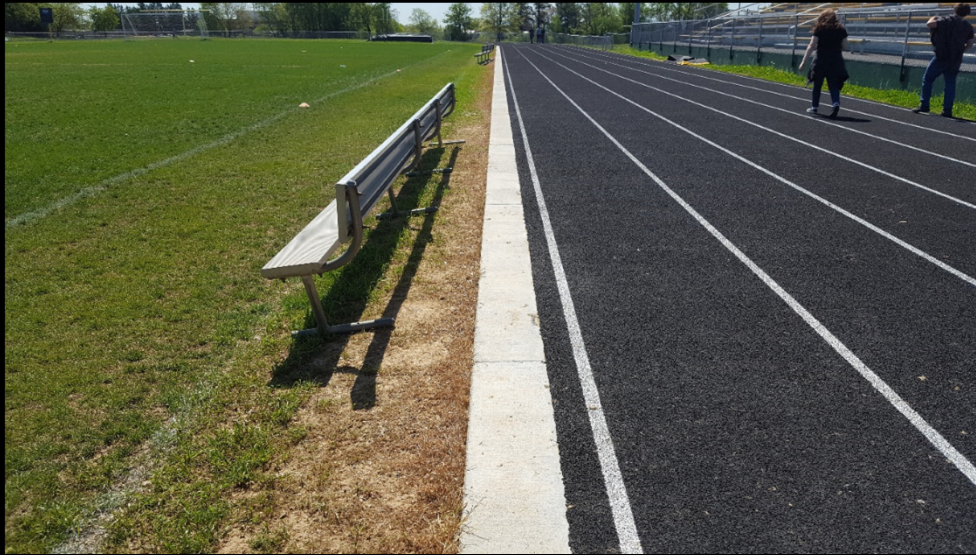
01. No Drain on Inside Perimeter and Elevation Change
