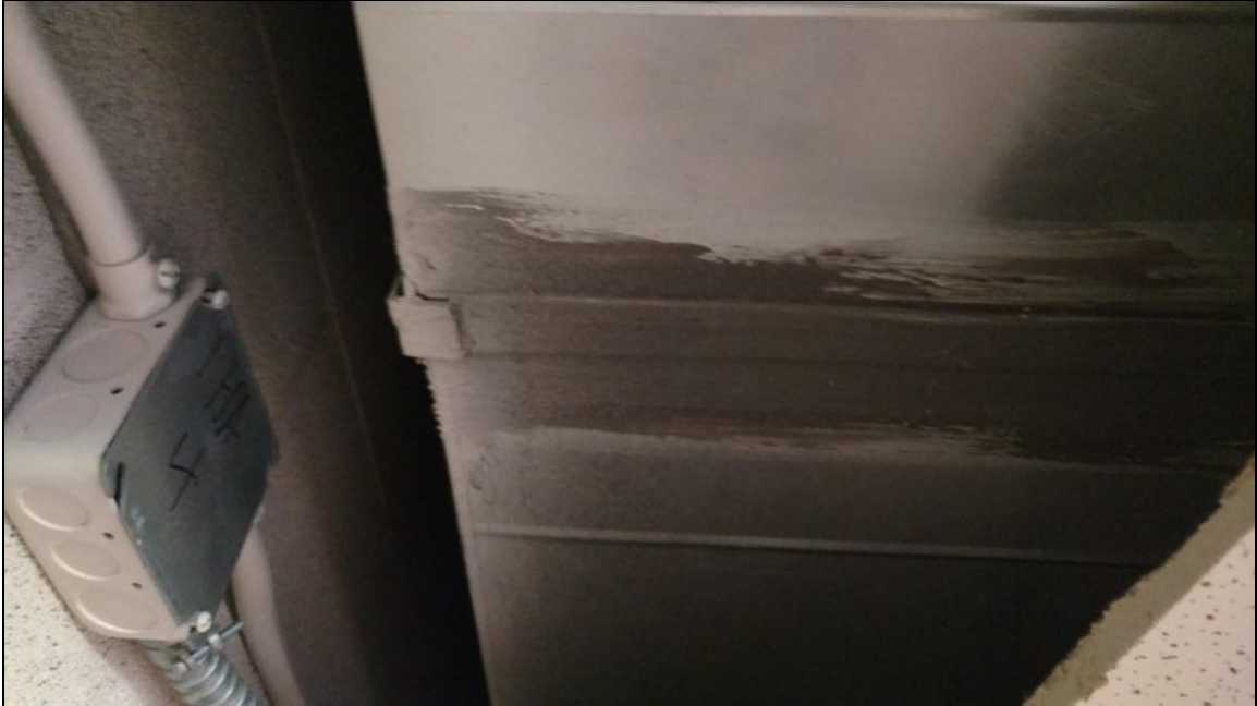
17 - View of typical grey HVAC duct mastic inside the school, homogeneous group 17
