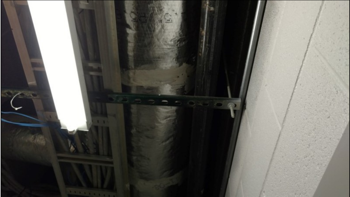
15 - View of typical white HVAC duct wrap mastic
