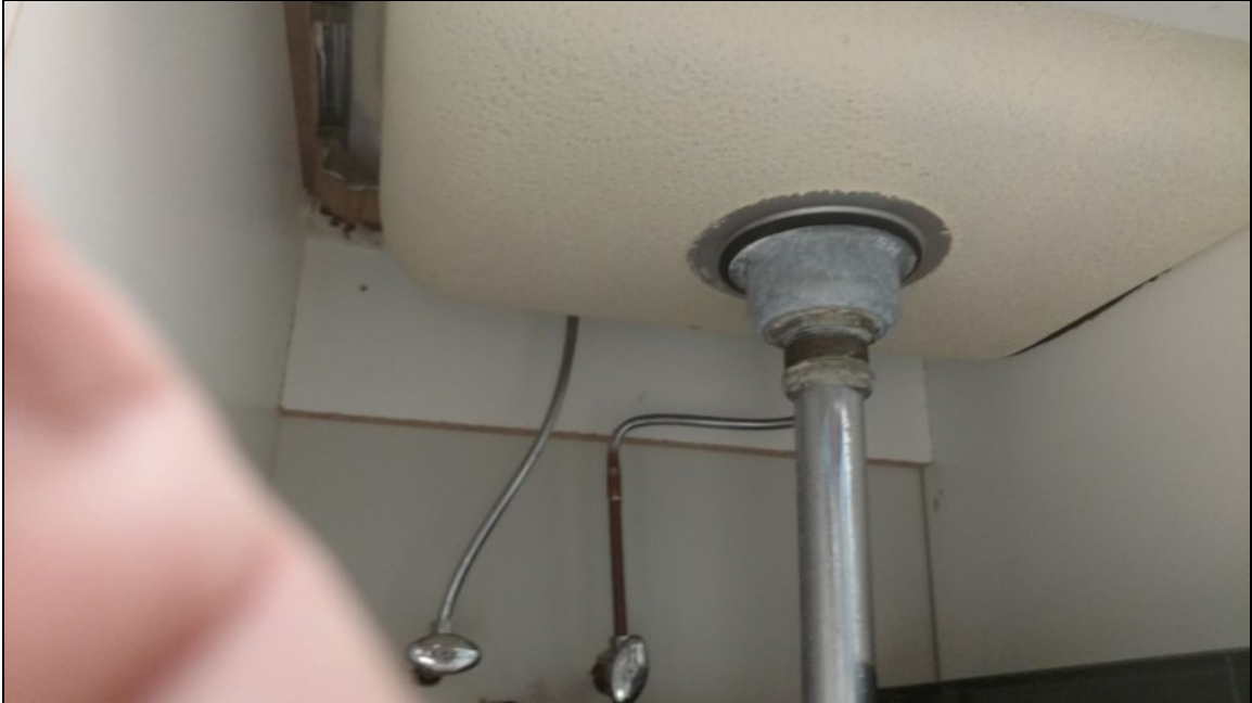
19 - View of typical white sink undercoating
