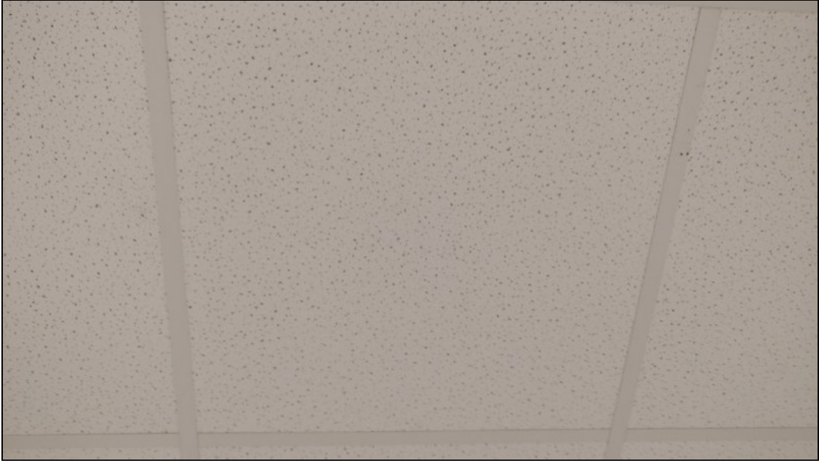
7 - View of typical pinhole/divot ceiling tile
