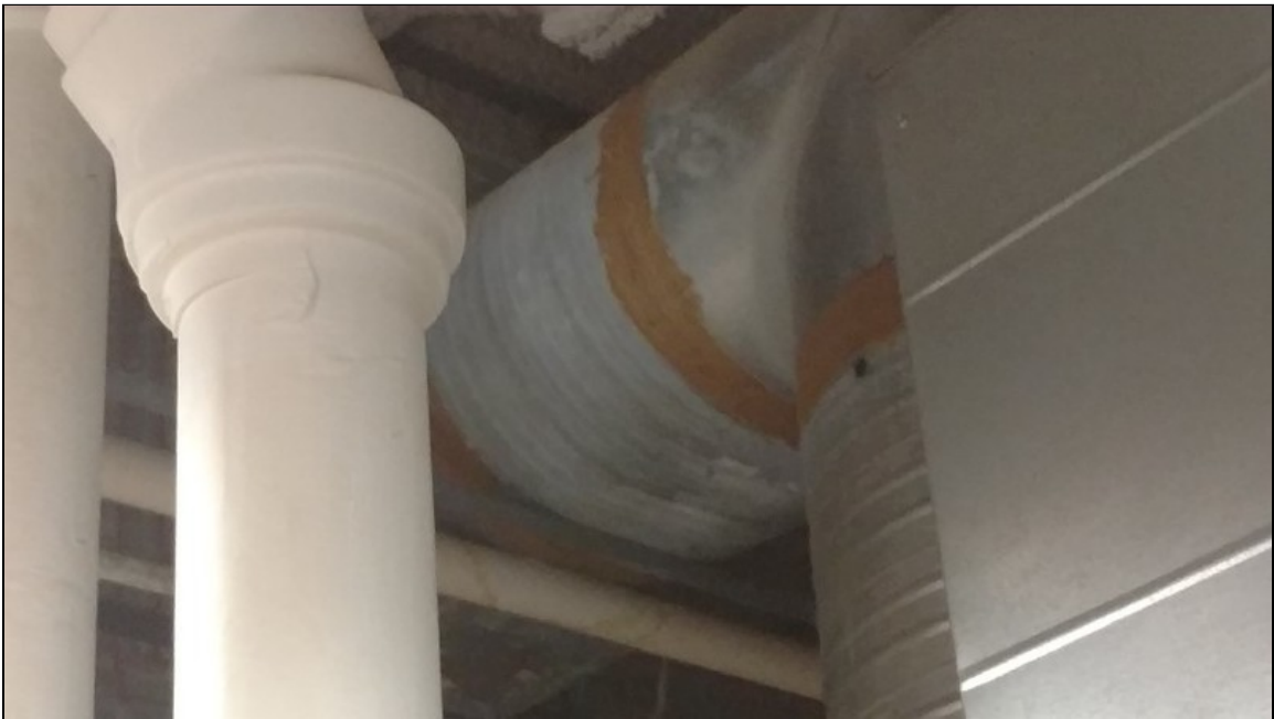
22 - View of typical brown HVAC duct mastic
