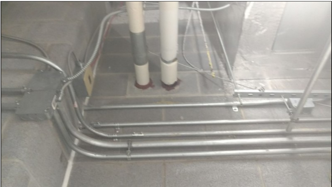
18 - View of typical red fire caulk
