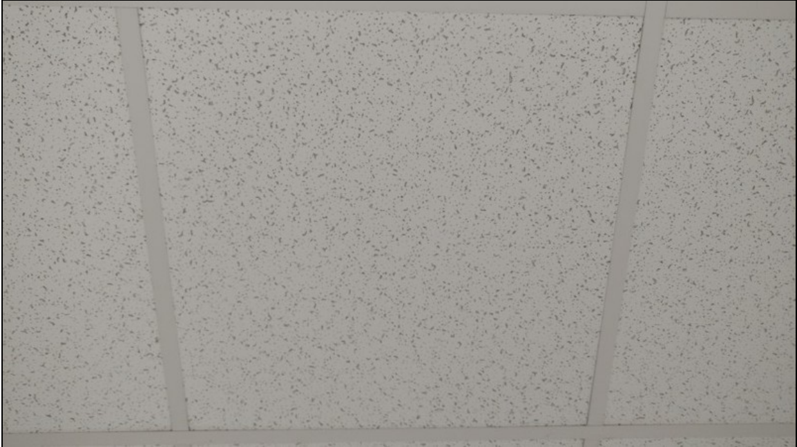
7 - View of typical fissure/pinhole ceiling tile
