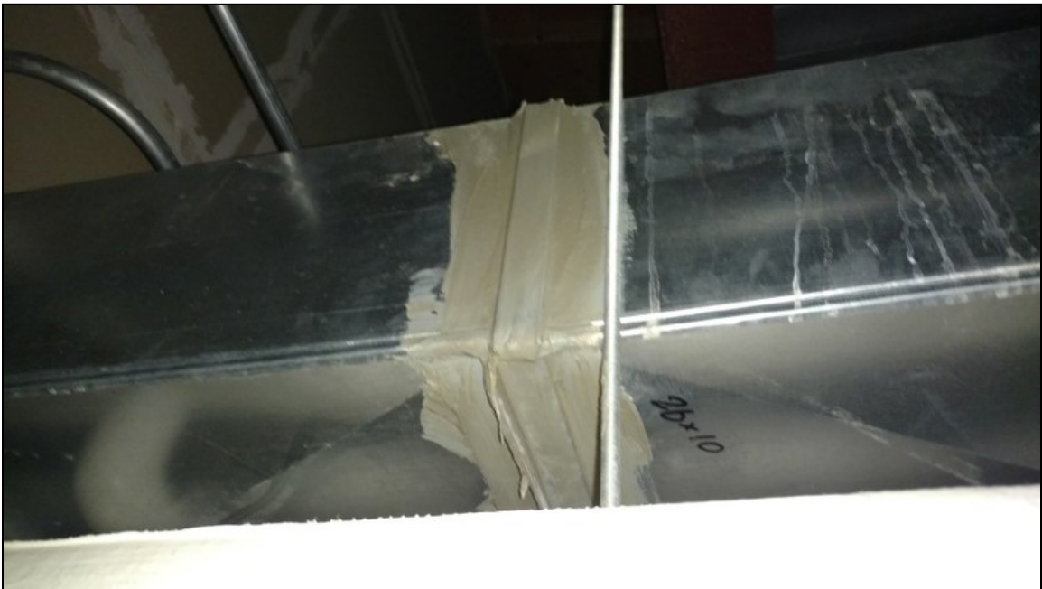
18 - View of typical grey HVAC duct mastic
