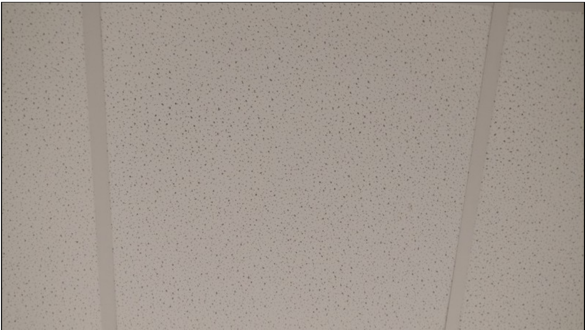
14 - View of typical pinhole ceiling tile
