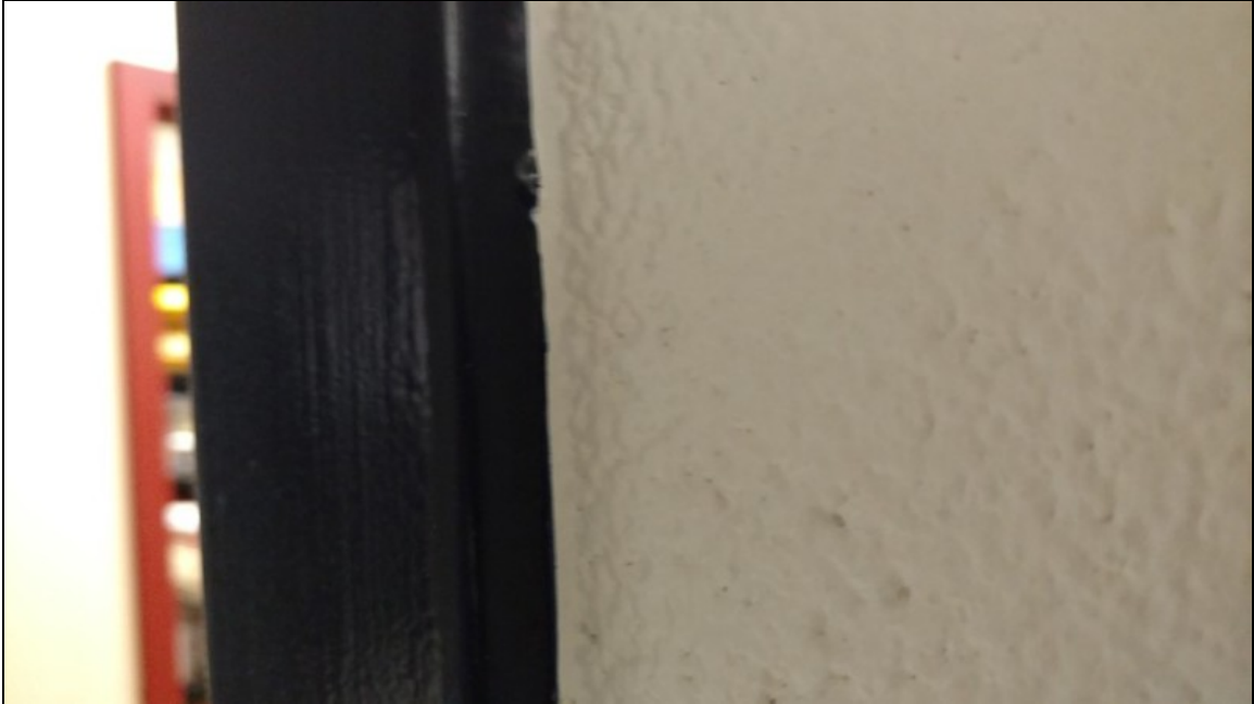
9 - View of typical interior metal door frame caulk
