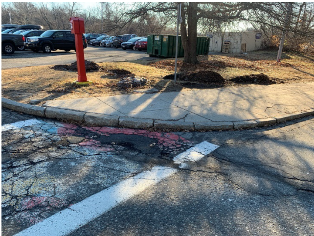
Missing Ramp at the end of Steve Miller Drive near the High School
