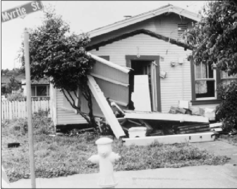
Houses that aren't bolted to their foundations shift off them.
