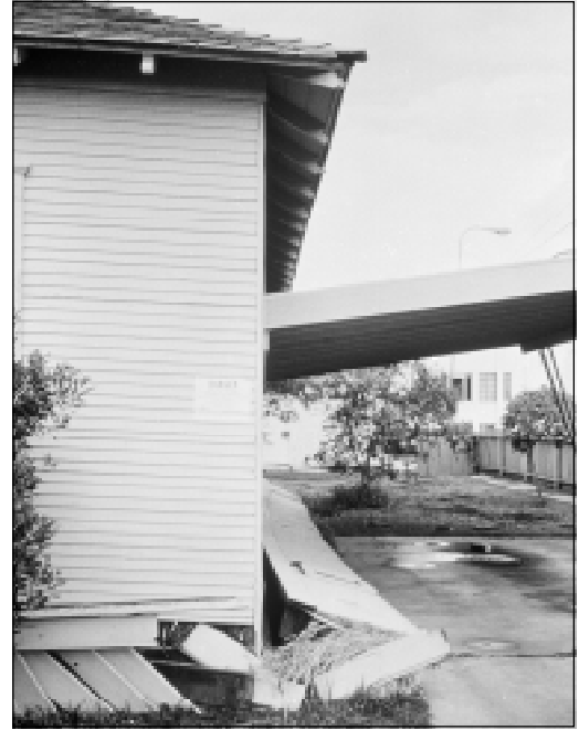
Unbraced cripple walls collapse.
