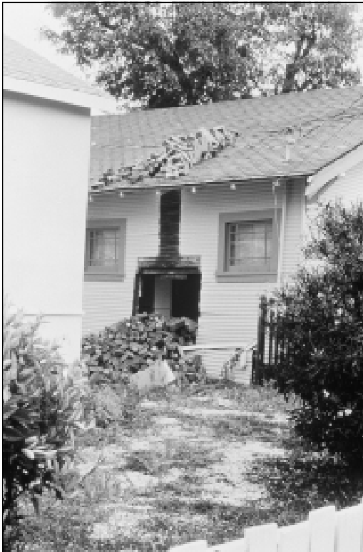
Chimney collapse is a widespread problem.
