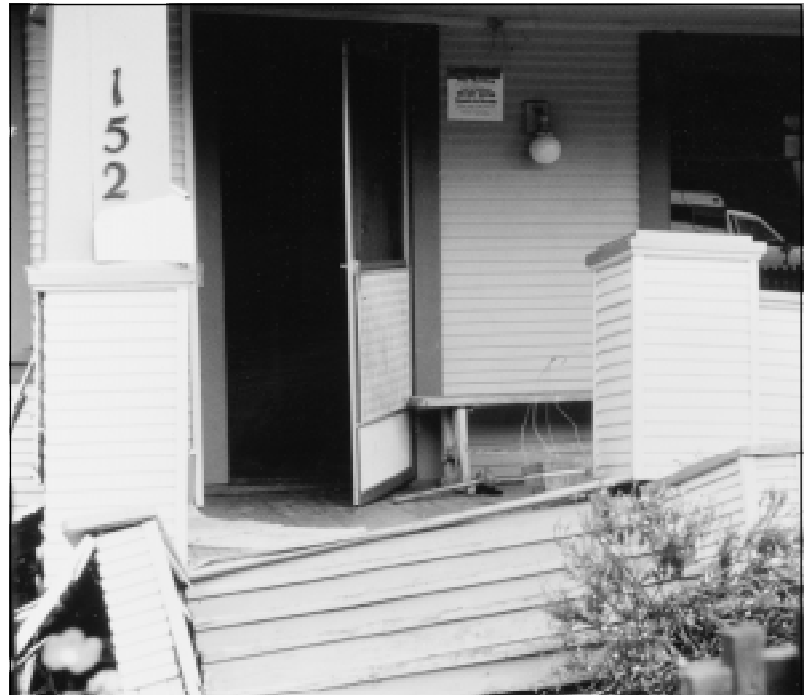
Porches and balconies can collapse if not properly attached.
