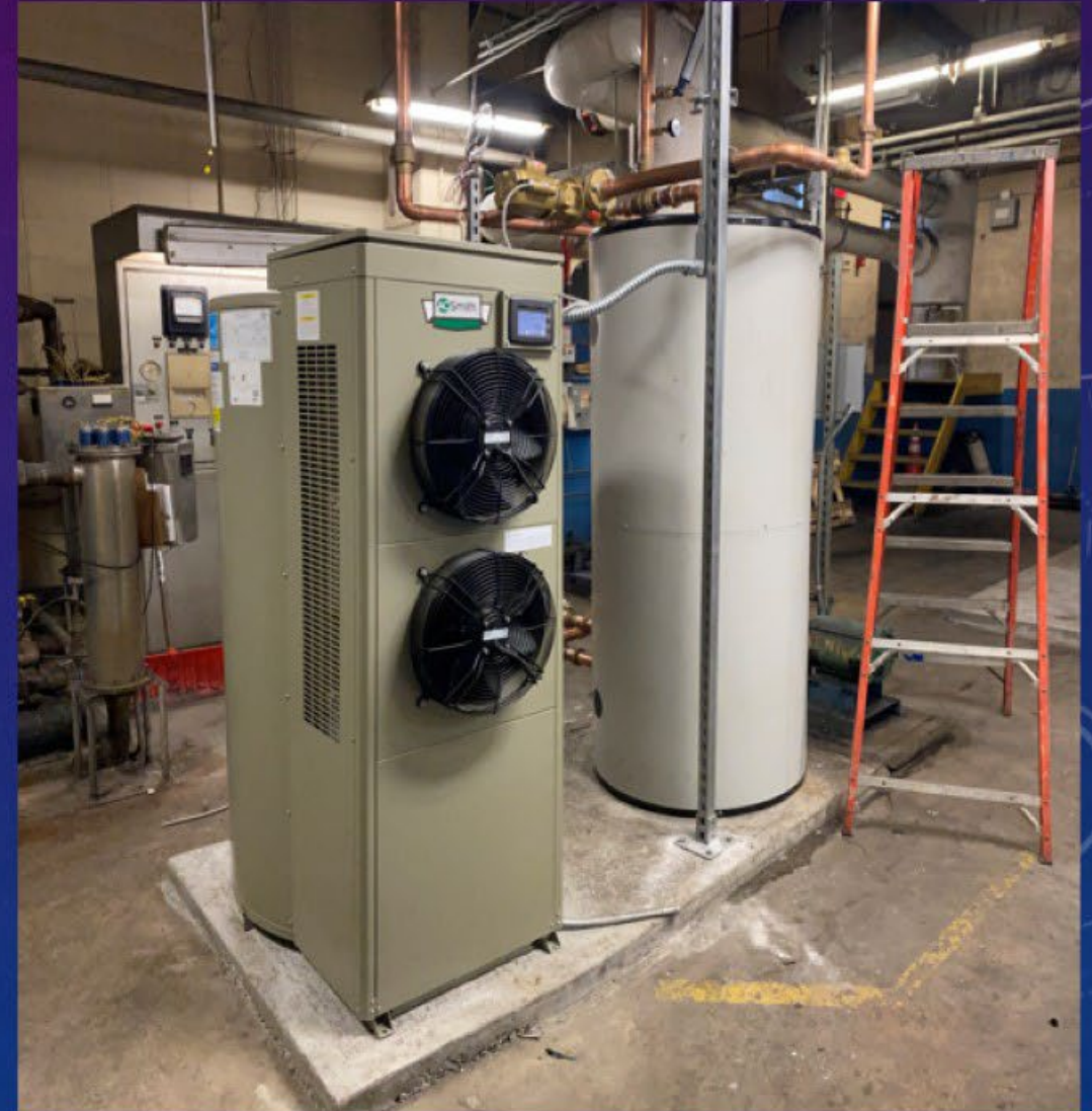
NEW HEATER & STORAGE TANK
