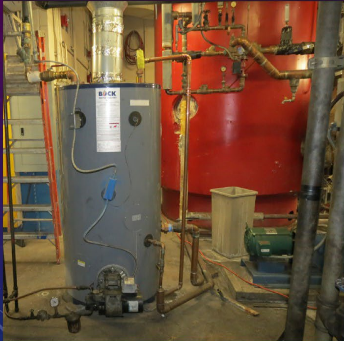
OLD HEATER & STORAGE TANK
