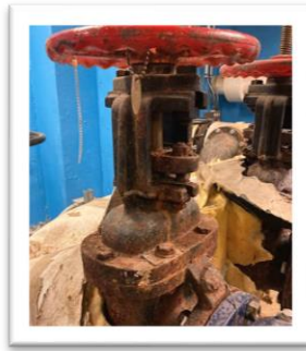
1970s water main valves
