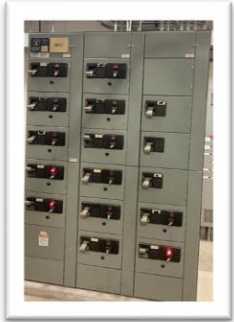
1962 Main Switch Gear
