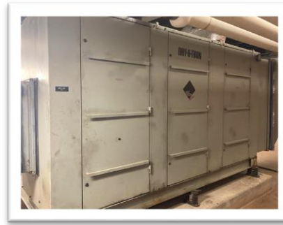
1988 Air Handling Unit
