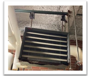
Rusted Housing of Heating Units
