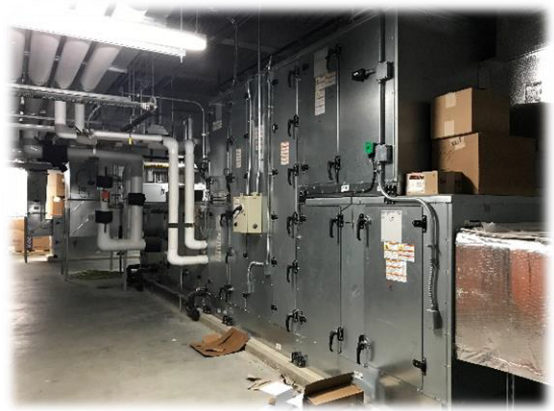
The air handler and water filling stations at Anna Mae Hays Elementary School are examples of the work needed to make the schools safer for students and staff during Covid and into the future.
