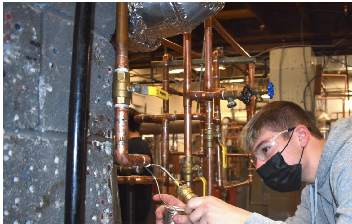
Wyatt Brown on the job as part of the PNW BOCES HVAC, Plumbing, and Pipe Fitting program.
