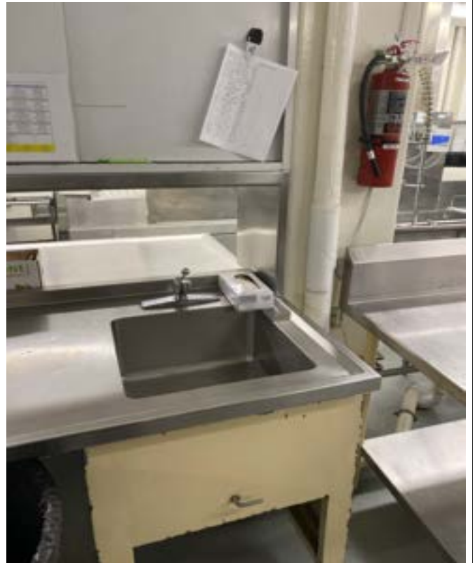
12/22/2023 - 5815-62 - Winnetonka High School - Kitchen-Middle Sink
