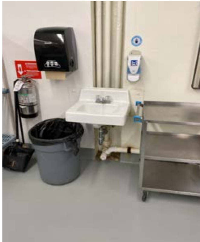
12/22/2023 - 5815-61 - Winnetonka High School - Kitchen-Northwest Handwashing Sink
