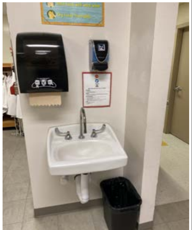
12/22/2023 - 5815-52 - Winnetonka High School - E4-West Handwashing Sink
