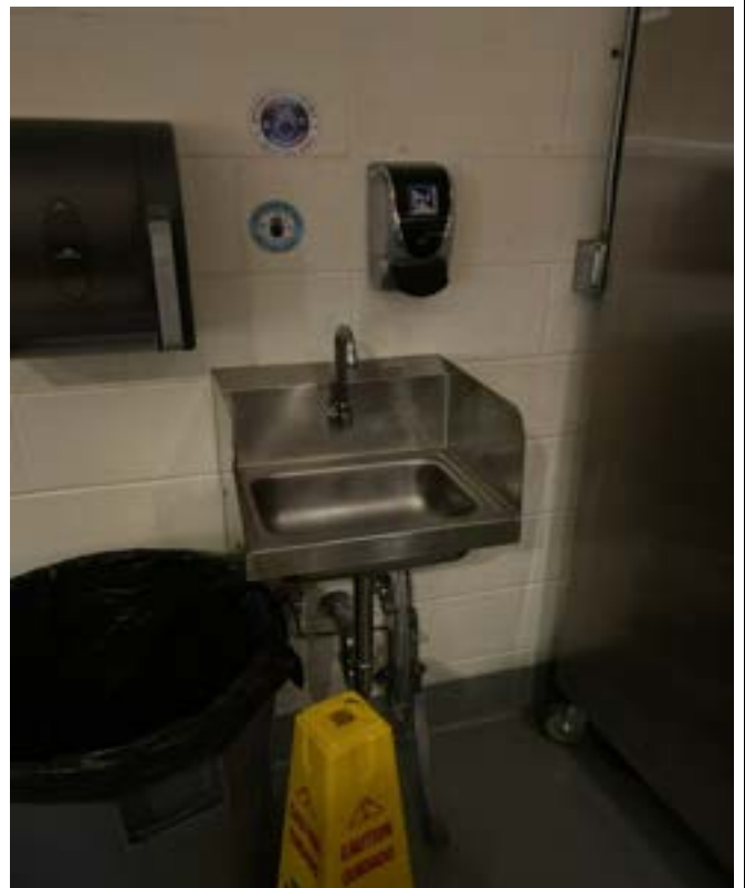
12/22/2023 - 5815-72 - Winnetonka High School - Serving-South Handwashing Sink
