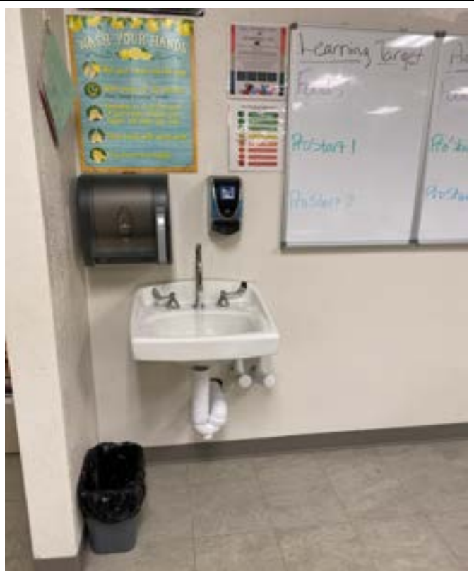
12/22/2023 - 5815-44 - Winnetonka High School - E4-North Handwashing Sink
