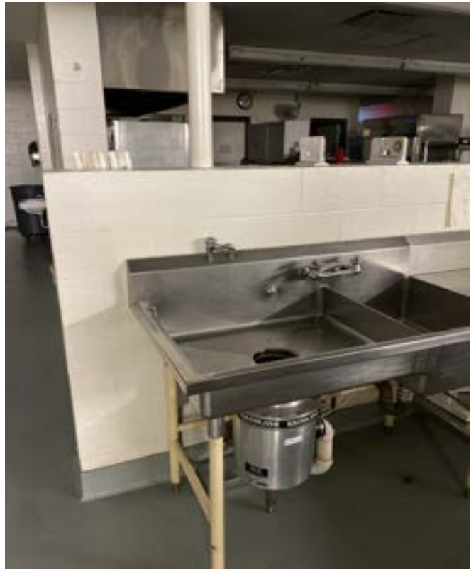
12/22/2023 - 5815-66 - Winnetonka High School - Kitchen-North Middle Sink by Fridge
