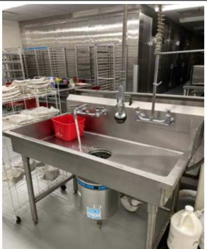
12/22/2023 - 5815-60 - Winnetonka High School - Kitchen-West Middle Sink
