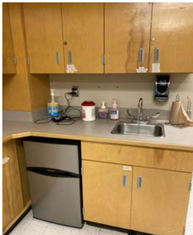
12/22/2023 - 5815-3 - Winnetonka High School - Nurse's Office-North Sink
