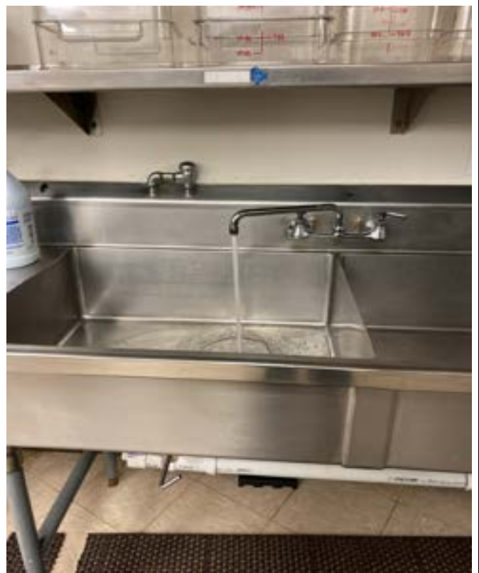
1/15/2024 - 1506-32 - West Englewood Elementary - Kitchen-Three Bay Sink-Left
