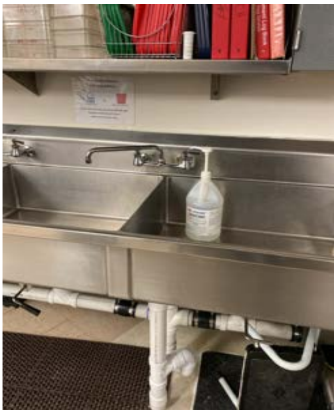
1/15/2024 - 1506-31 - West Englewood Elementary - Kitchen-Three Bay Sink-Right
