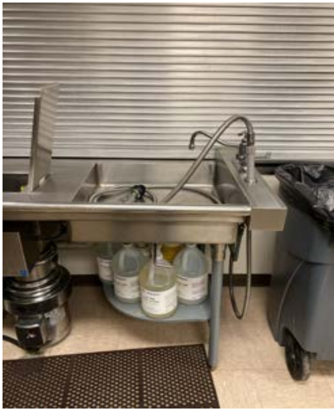
1/15/2024 - 1506-29 - West Englewood Elementary - Kitchen-Closest to Cafe
