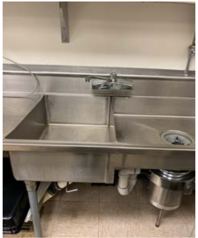
1/15/2024 - 1506-34 - West Englewood Elementary - Kitchen-Southwest Sink
