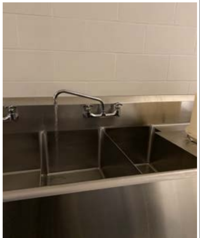
1/8/2024 - 7301-36 - Rising Hill Elementary - Kitchen-Three Bay Sink-Right
