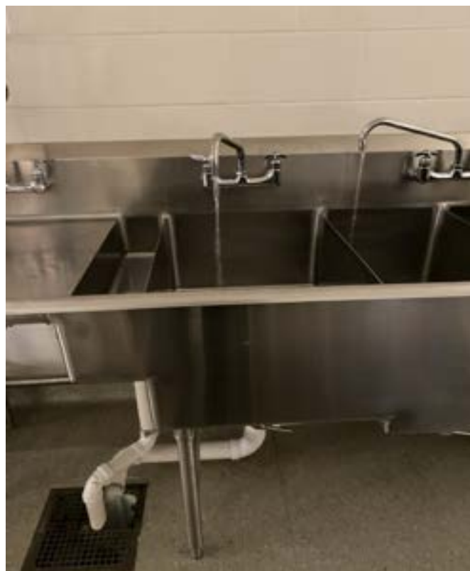
1/8/2024 - 7301-35 - Rising Hill Elementary - Kitchen-Three Bay Sink-Left
