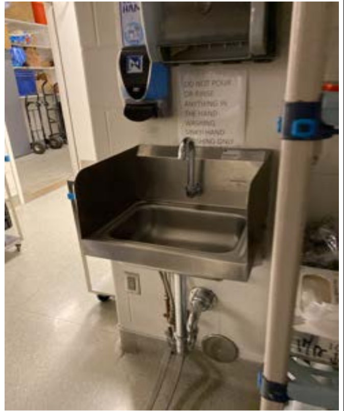
1/8/2024 - 7301-34 - Rising Hill Elementary - Kitchen-Northwest Handwashing Sink
