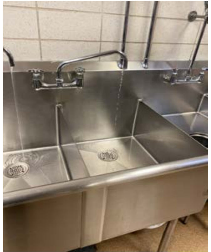
1/23/2024 - 5900-18 - Oakwood Manor - Kitchen- Four Bay Sink-Middle
