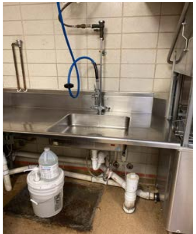
1/23/2024 - 5900-20 - Oakwood Manor - Kitchen- Northeast Sink
