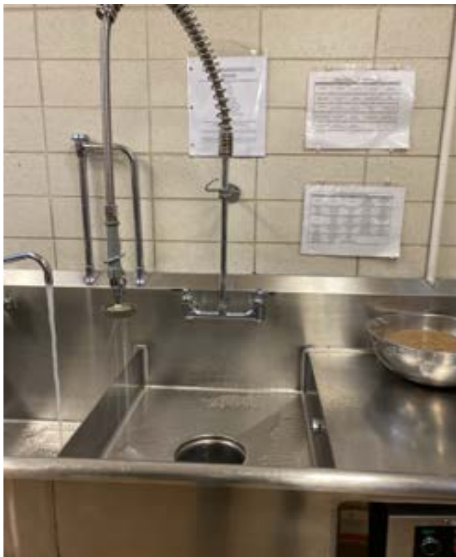
1/23/2024 - 5900-19 - Oakwood Manor - Kitchen- Four Bay Sink-Right
