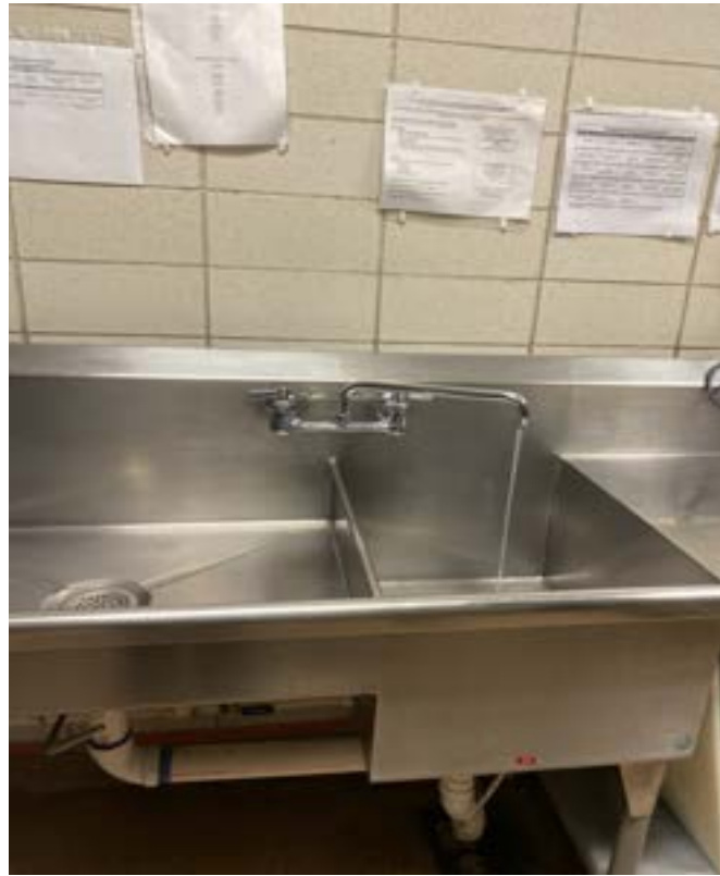
1/23/2024 - 5900-21 - Oakwood Manor - Kitchen- South Sink
