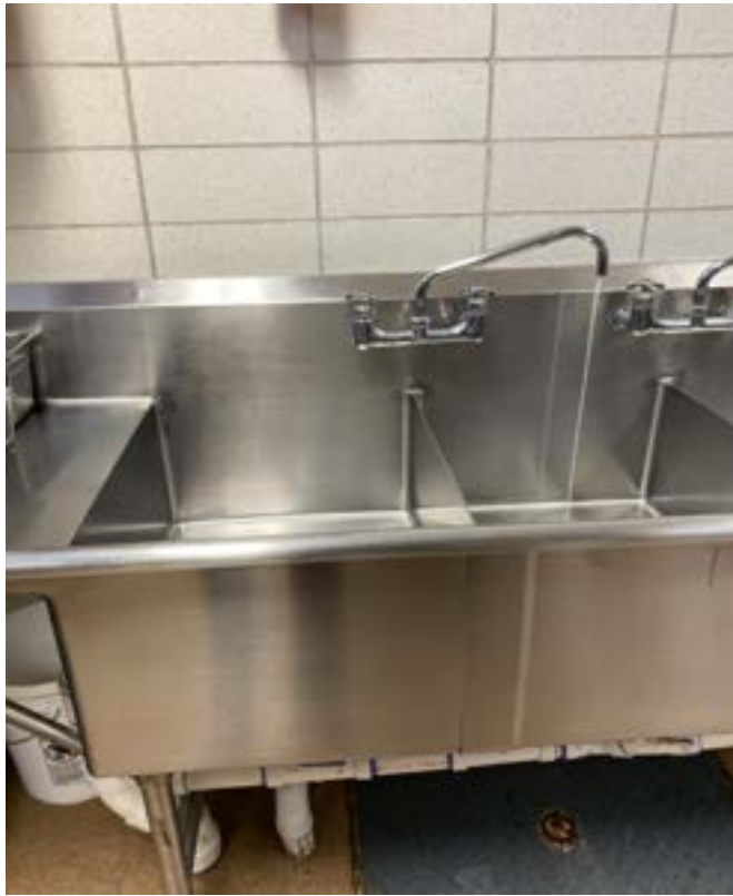
1/23/2024 - 5900-17 - Oakwood Manor - Kitchen- Four Bay Sink-Left
