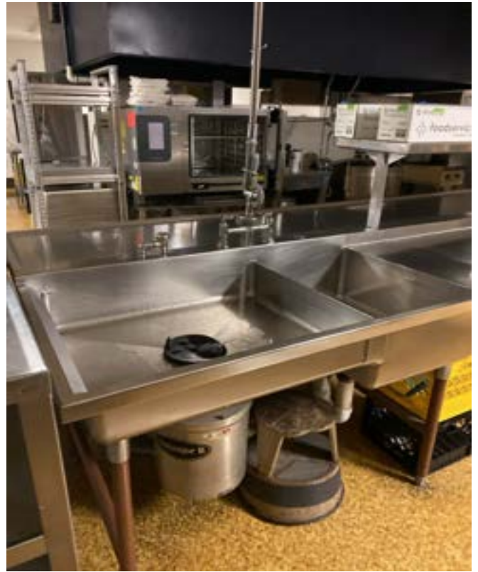
1/15/2024 - 515-50 - New Mark Middle School - Kitchen-Middle by Steam Kettle
