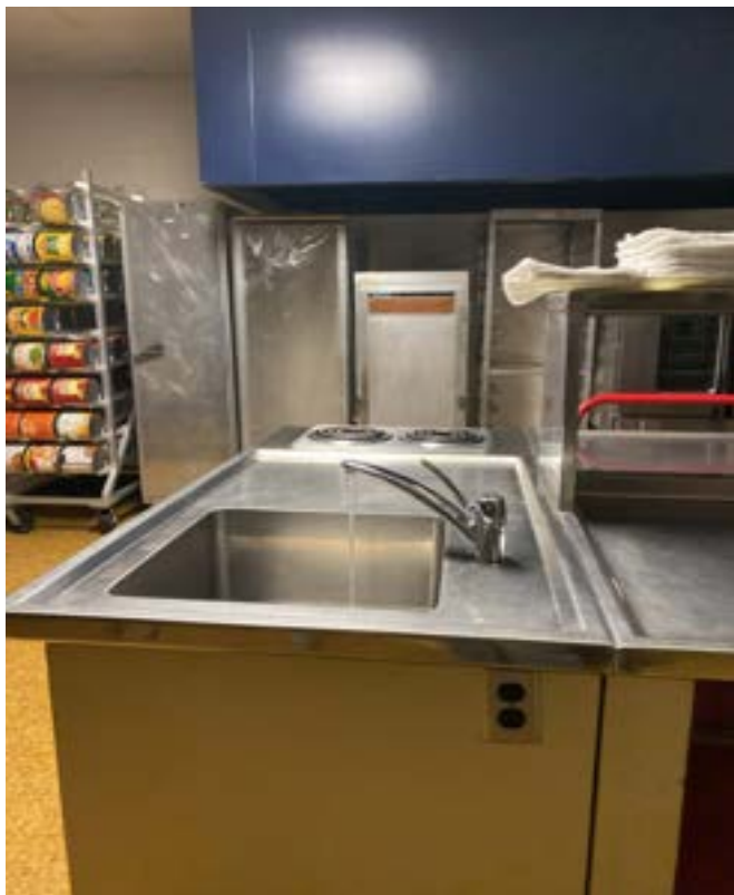
1/15/2024 - 515-51 - New Mark Middle School - Kitchen-North Middle Sink
