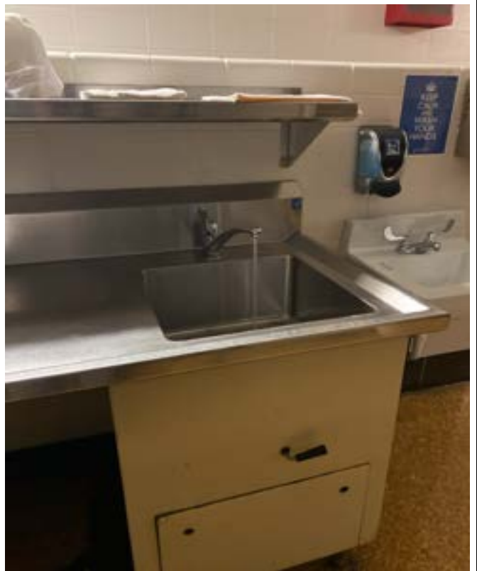
1/15/2024 - 515-48 - New Mark Middle School - Kitchen-South Middle Sink
