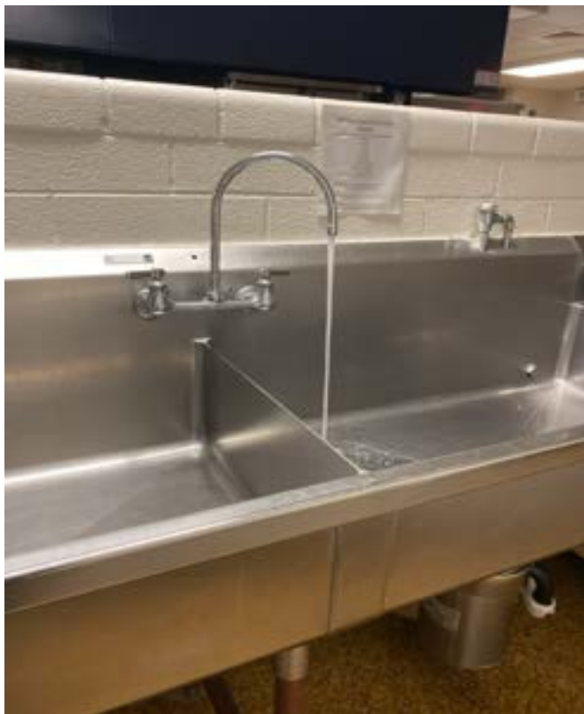
1/15/2024 - 515-47 - New Mark Middle School - Kitchen-Three Bay Sink-Right
