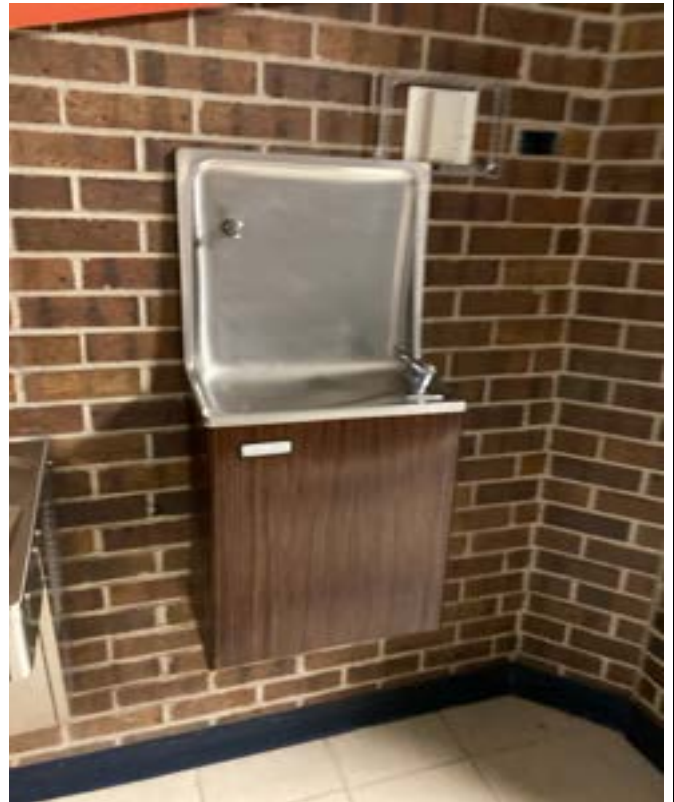
1/15/2024 - 515-58 - New Mark Middle School - Commons-Right
