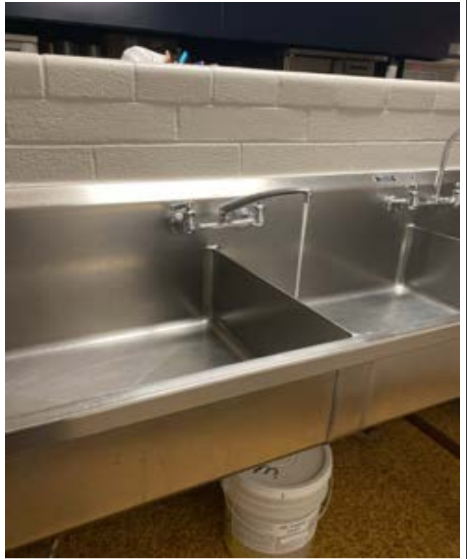
1/15/2024 - 515-46 - New Mark Middle School - Kitchen-Three Bay Sink-Left
