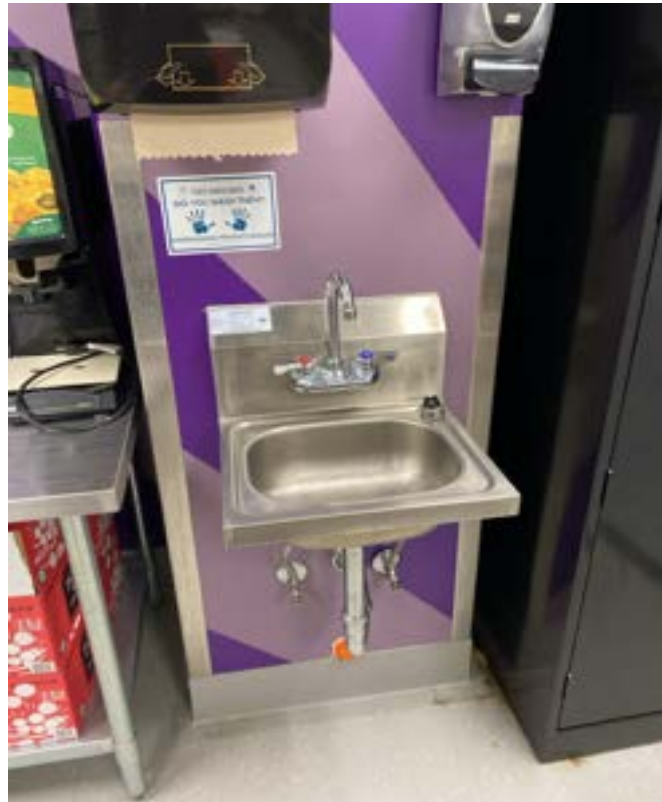
12/21/2023 - 620-73 - NKC High School - Concessions-Handwashing Sink
