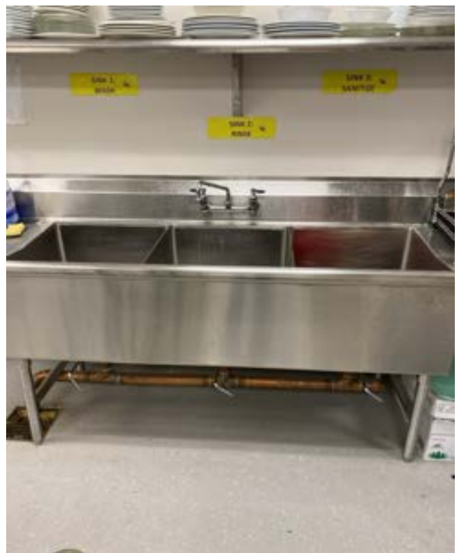
12/21/2023 - 620-48 - NKC High School - B143-Three Bay Sink
