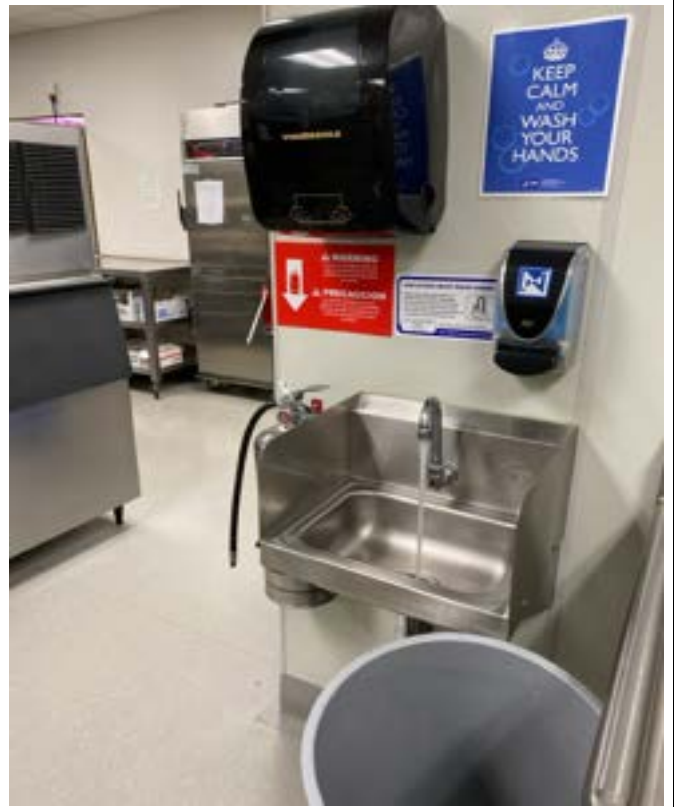
12/21/2023 - 620-62 - NKC High School - Kitchen- Handwashing by Ice Machine
