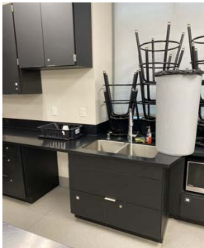
12/21/2023 - 620-55 - NKC High School - B145- Southeast Sink
