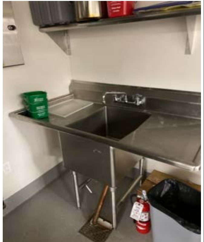
12/21/2023 - 620-50 - NKC High School - B143- Next to Oven
