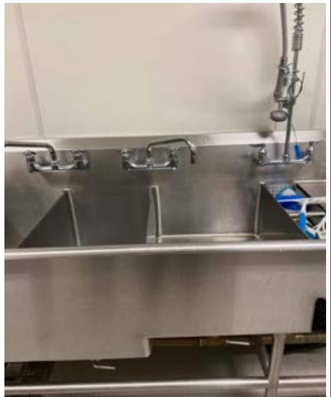
12/21/2023 - 620-64 - NKC High School - Kitchen- Three Bay Sink-Middle
