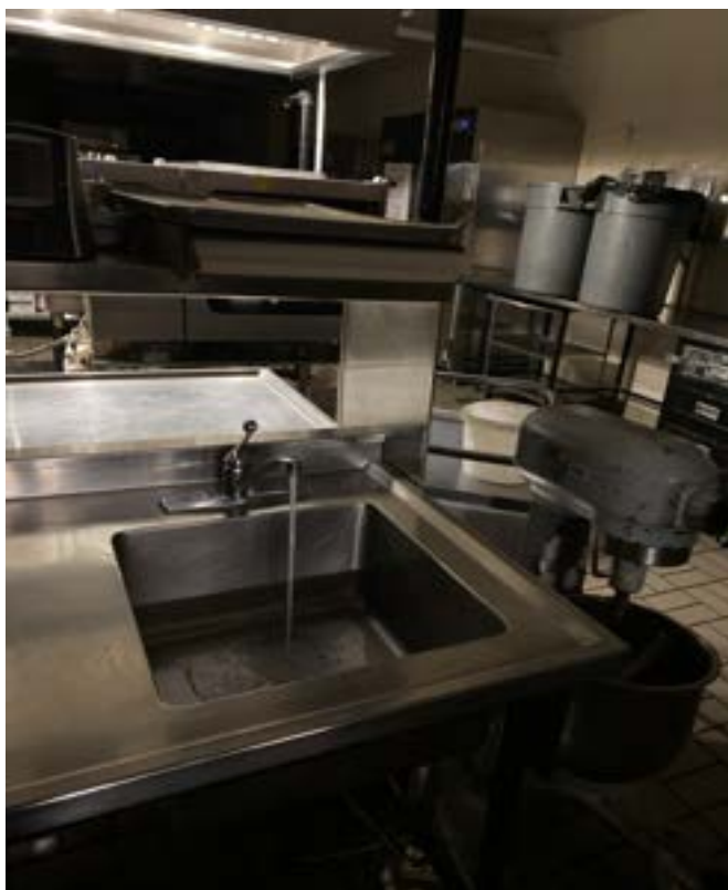
12/26/2023 - 825-51 - Oak Park High School - Kitchen-South Middle Sink
