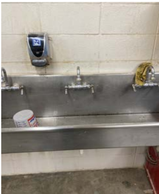
12/26/2023 - 825-43 - Oak Park High School - C121-Right Sink-Middle
