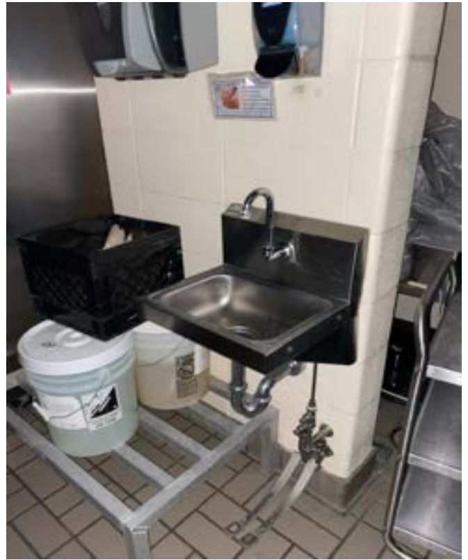
12/26/2023 - 825-58 - Oak Park High School - Kitchen-North Handwashing Sink
