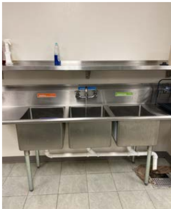
12/26/2023 - 825-23 - Oak Park High School - F113-3 Bay Sink
