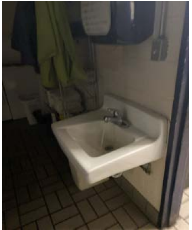
12/26/2023 - 825-50 - Oak Park High School - Kitchen-South Handwashing Sink
